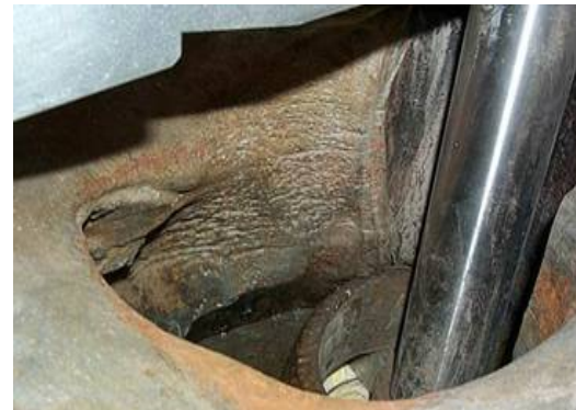
Davis Besse (March 2002): CRDM penetration and head wastage
