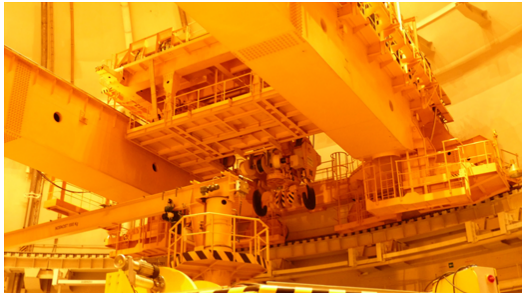
Polar crane in reactor hall as tool for measurement of core shroud dimension
