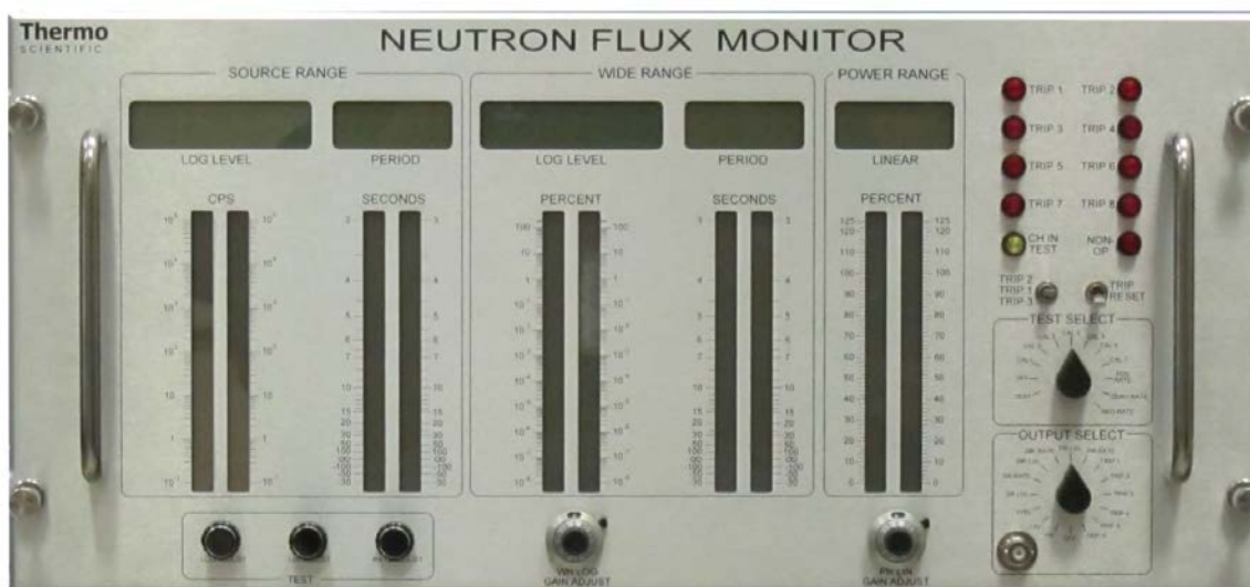
Figure 7.5 - Wide Range Log Period Power Module (PPM)
