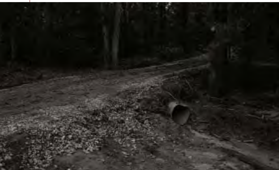
Figure 1. A well located, constructed and maintained system of forest roads will be safer, allow longer operating periods, and reduce operating and maintenance costs.
