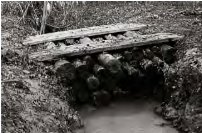
Figure 10. Temporary bridges and crossing structures should be removed when no longer needed for timber harvesting operations.
