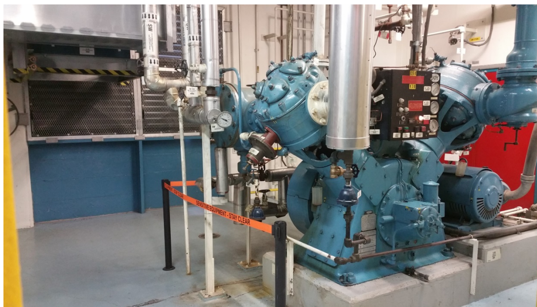
Figure 5-4: Example Air Compressor with Subcomponents
