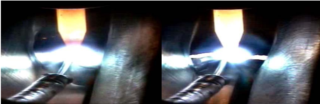
Figure 3-12. Photo sequence captured from VIDs showing differences in root gap width as the weld bead progressed clockwise around the circumference. The shell wall is on the right side of the photo and the cover plate is on the left. The VID camera is mounted to view the front of the arc.
