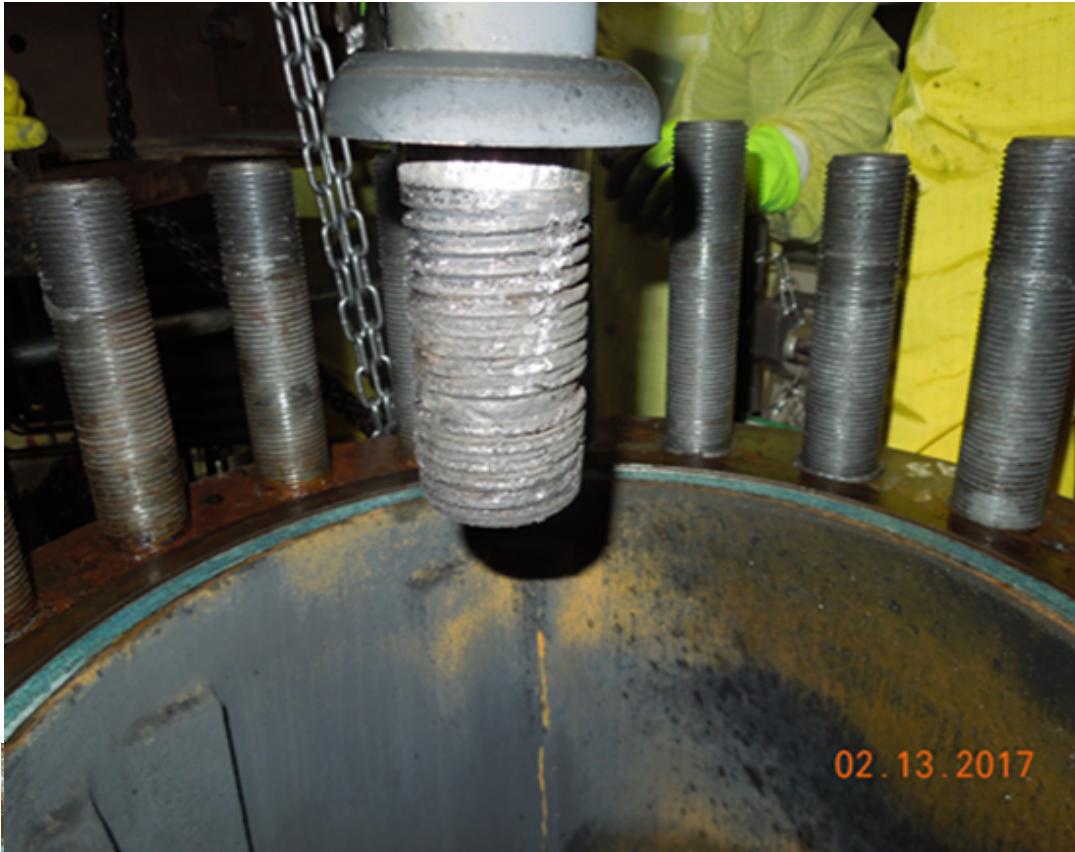
Figure: As Found Pictures of Failed Unit 2 HPCS Injection Valve Stem to Wedge Connection
