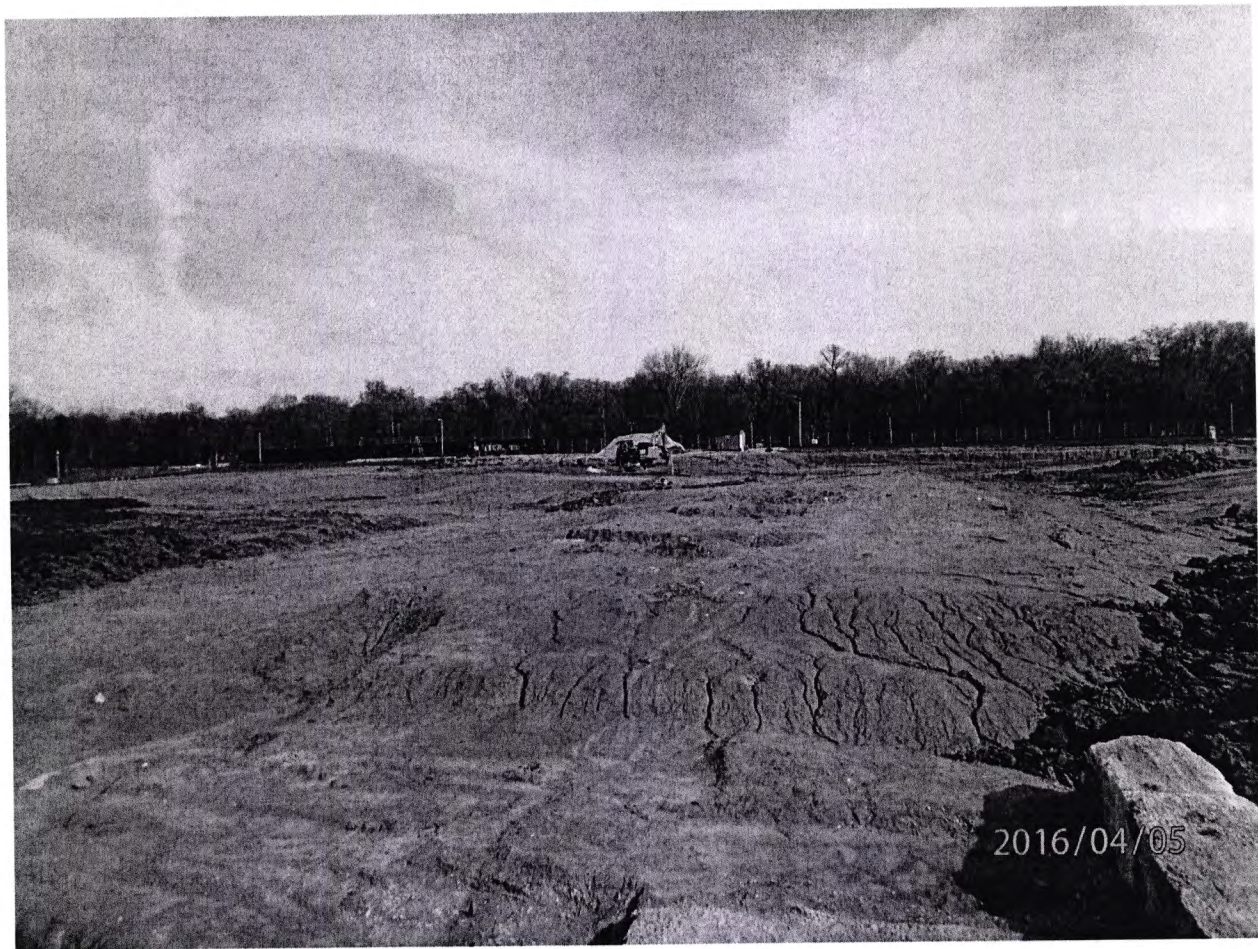
LSA 08-03 in the foreground 04/05/2016 the day prior to Pre-backfill Confirmatory GWS conducted on 04/06/2016.
