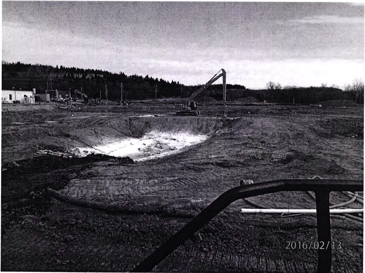
Application of Catalyzed Persulfate in LSA 08-02 completed using extended arm excavator for work safety. Bags remain in excavation to minimize exposure to workers.
