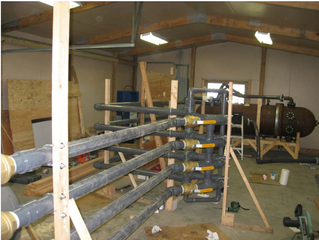
Figure 2. Photographs of the steam delivery system at nominal one-eighth scale. (Ref. 1).
