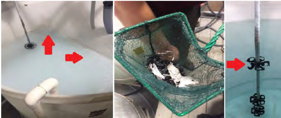
Photo 4 – Issue with calcium phosphate tank – additional debris found, as a result, of contact between the mixing-propeller and the tank lid
