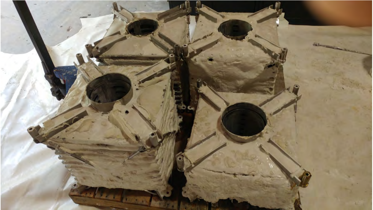
Photo 9 – Entire strainer stack showing most of strainer engulfed in debris
