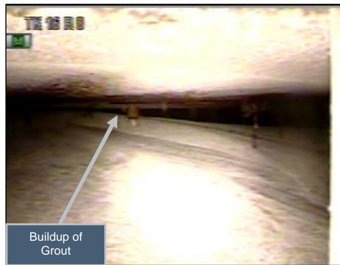
Figure 3.2-3: Uneven Buildup (i.e., mounding) of Grout under Riser 6 near the End of Lift 5
