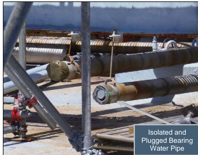
Figure 3.1-1: Tank 16 Bearing Water Pipe Isolated
