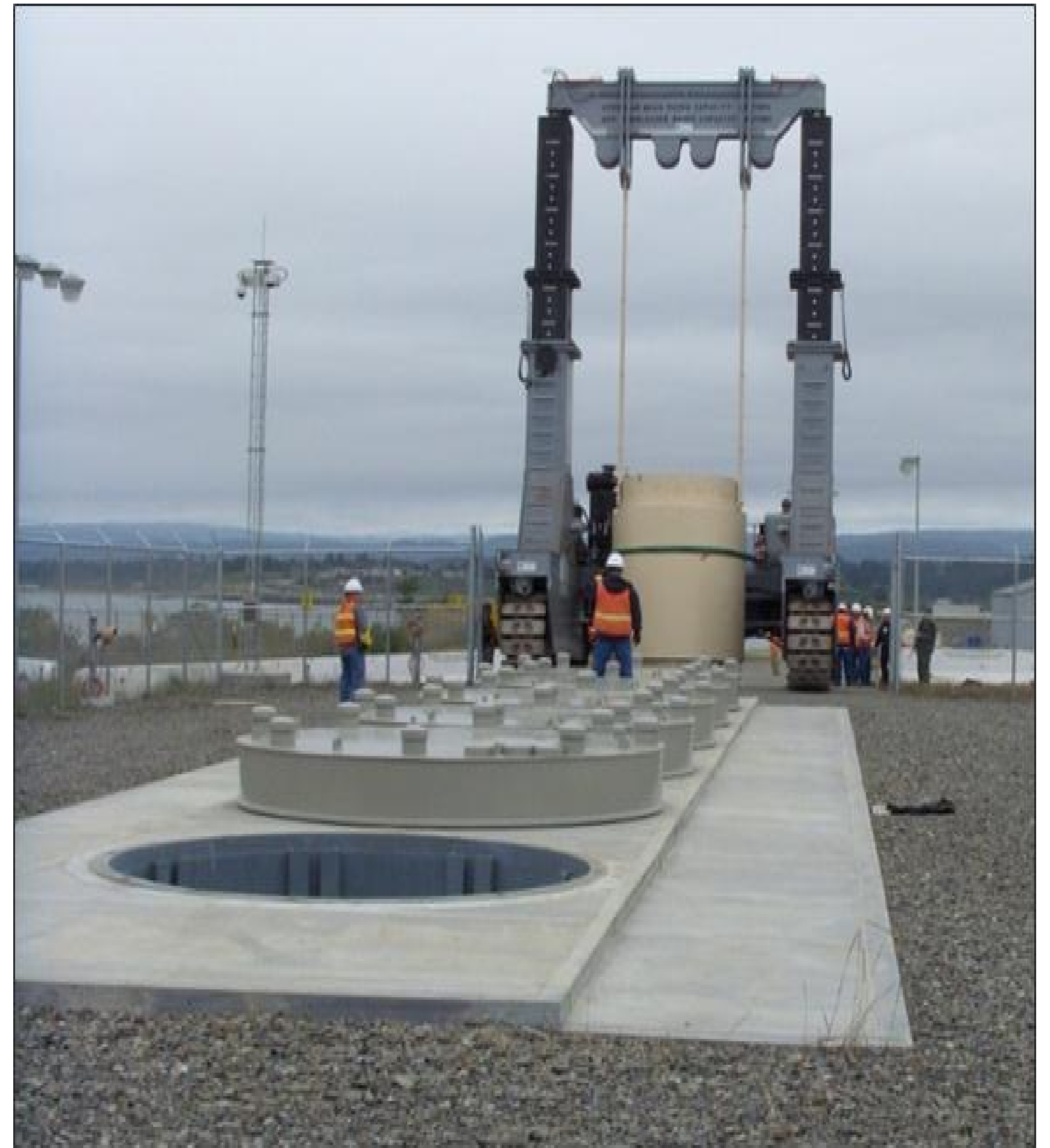
Below-grade Storage at Humboldt Bay Power Plant, in Eureka, CA
