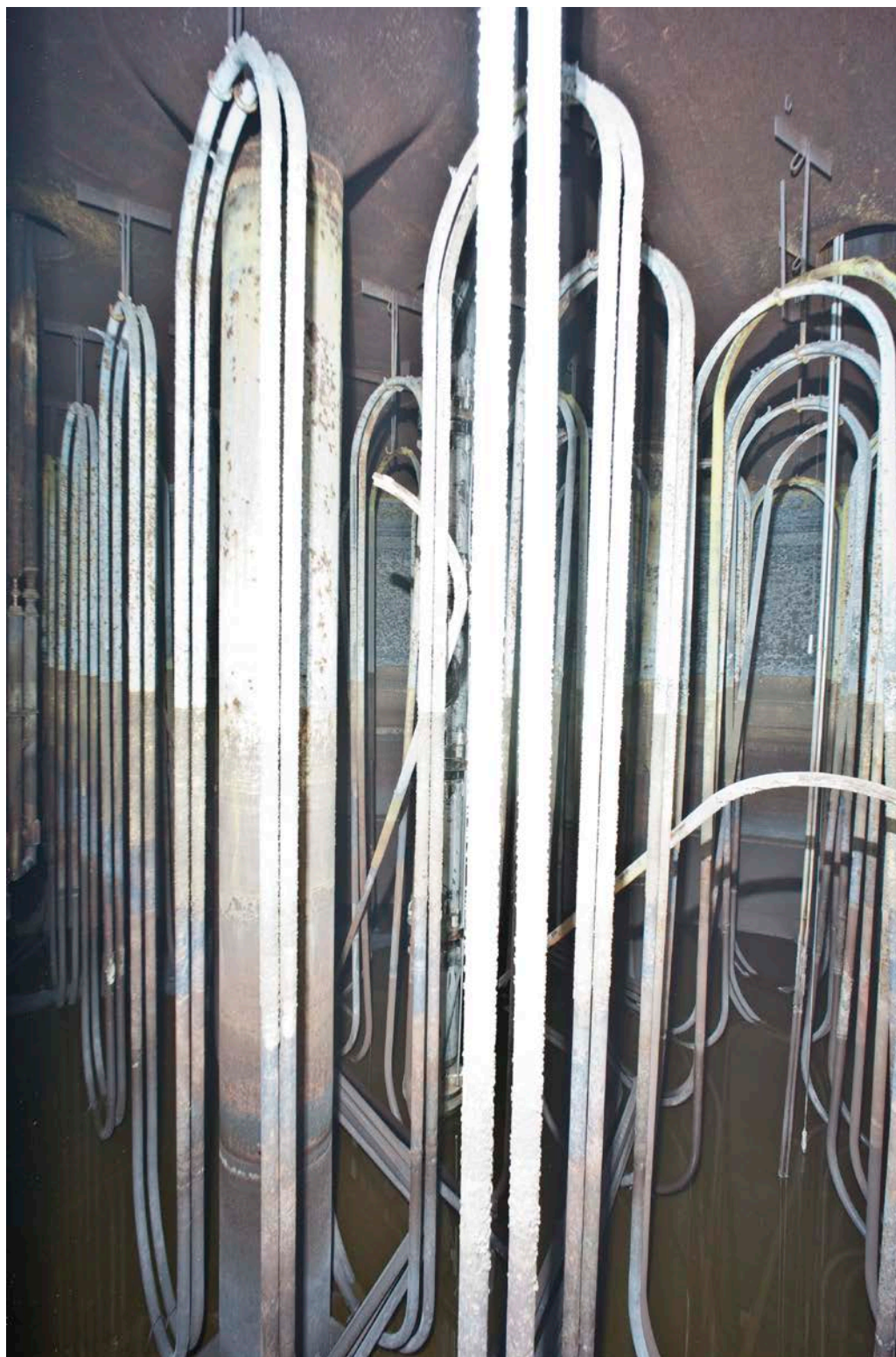
Figure 1: Tank 12 Guillotined and Broken CCW Coils
