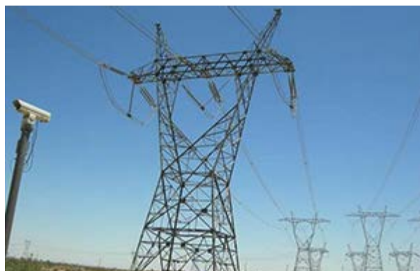
Regulated High Voltage Transmission Lines, 1,296 MW (Mead Adelanto), 1,900 MW (Mead Phoenix)
