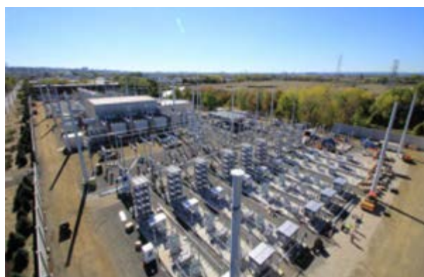
Underground / Sub-sea Trans, 660 MW
