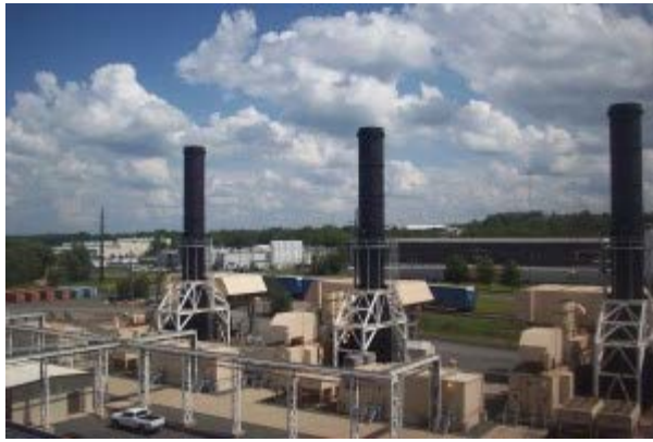
Hazleton Facility, PA
