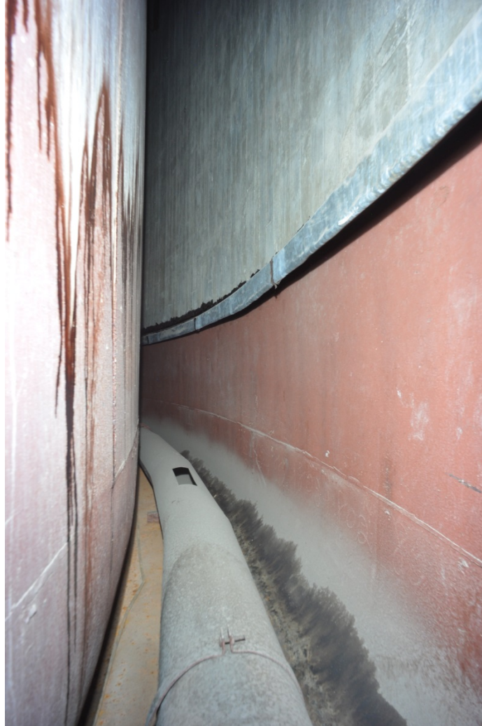
Figure 6.2.1.1: View of Tank 12H Annulus and Horizontal Ventilation Duct (West Riser, September 2012)
