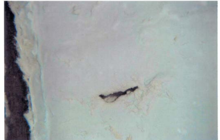
Picture 30: Underwater picture of breakthrough
