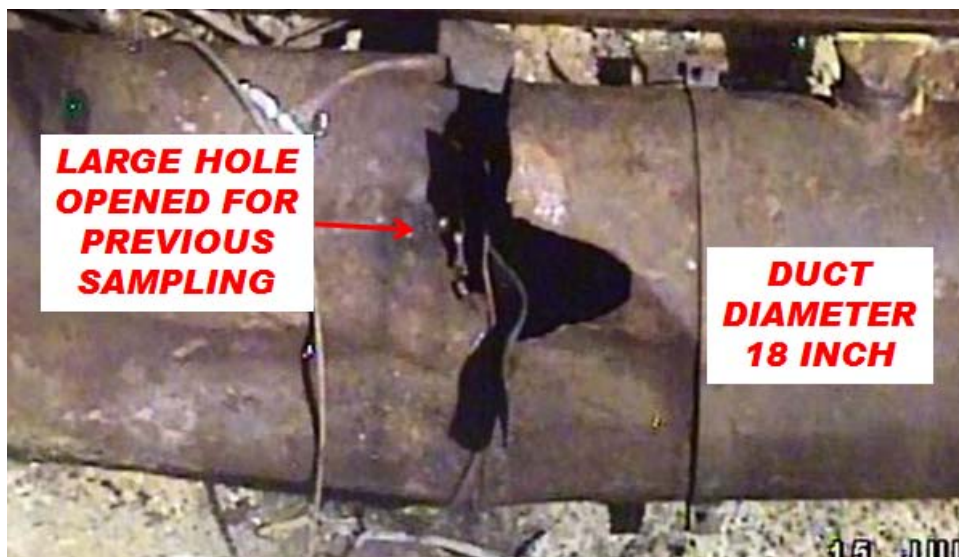
Figure 18: (Area at STA 0+00 measured at 5.25 inches. Photo A U-ESR-H-00113)
