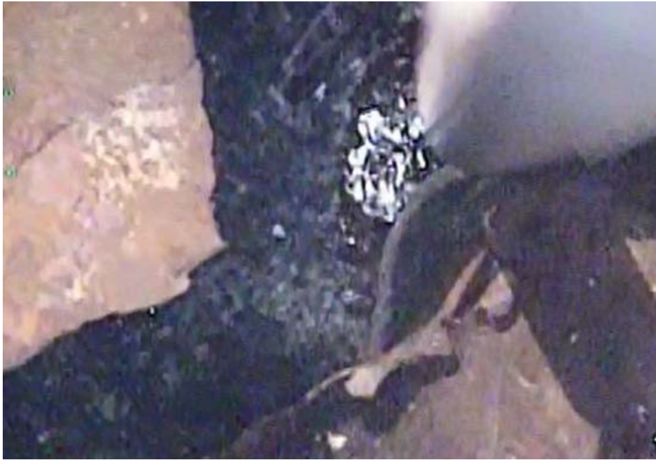
Figure 12: (Area at STA 0+00. Photo B U-ESR-H-00113)
