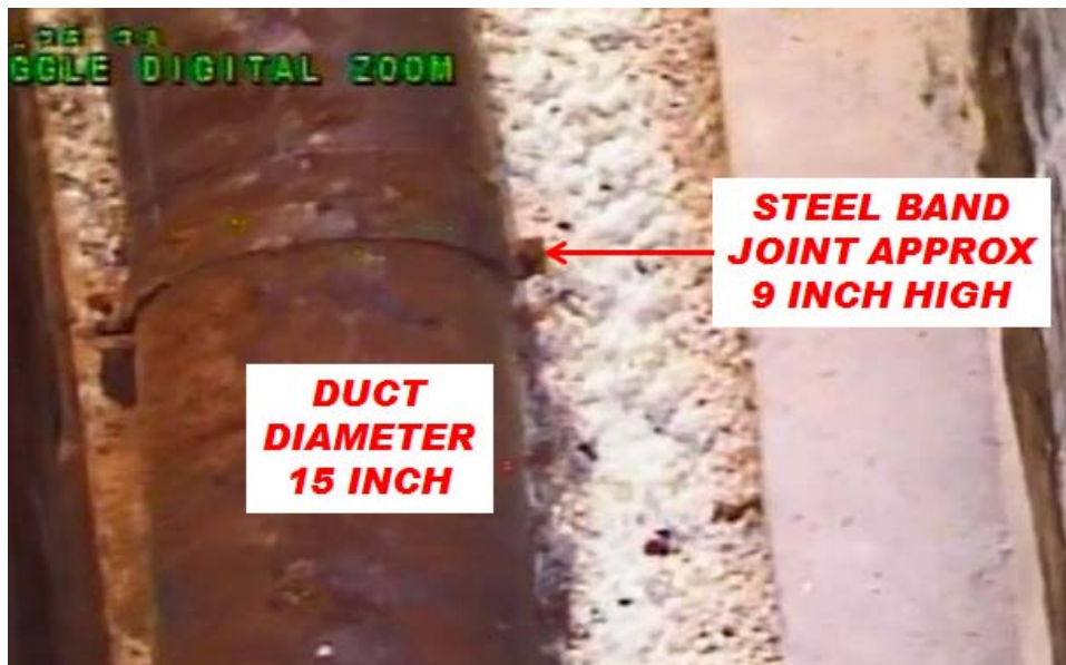
Figure 8: (Area at STA 3+00 near STA 3+50 measured at 3 inches. Photo F U-ESR-H-00113)
