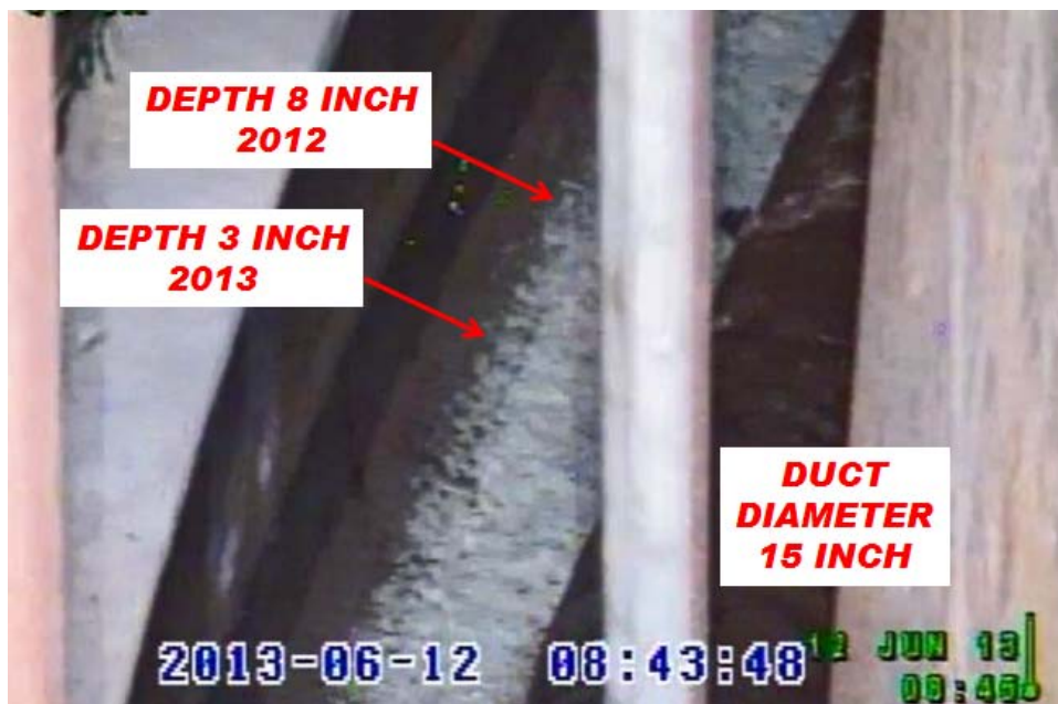
Figure 3: (Area at STA 5+00 interpolated to a height of 3 inches in 2013. Photo I U-ESR-H-00113)
