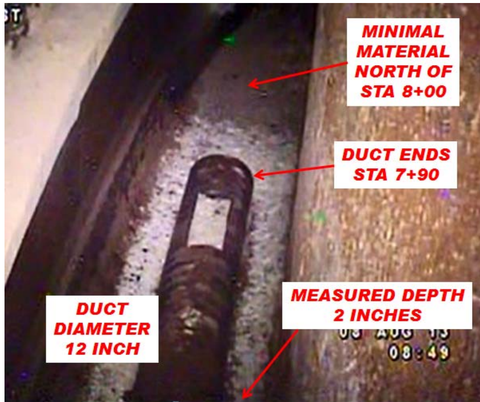
Figure 9: (Area at STA 8+00 near STA 7+00 measured at 2 inches. Photo L U-ESR-H-00113)
