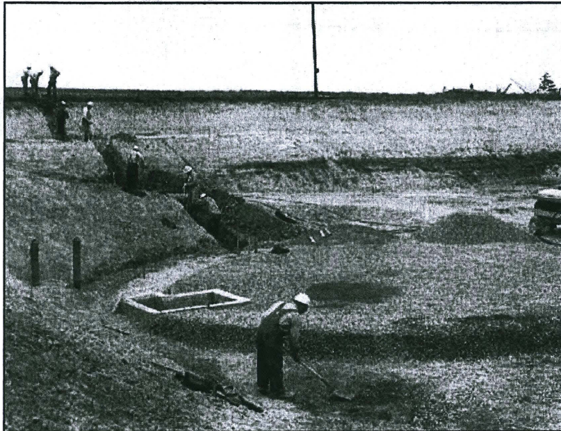
Figure 5. Fuel Oil Storage Tank Unit 2 Under Construction (May 25, 1955) This is the Location of Alternative S-2 for the Current Project
