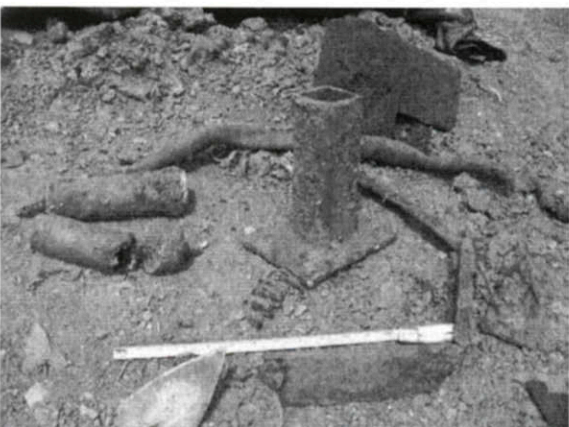
Photo #: PGE Decommission IF-4 View: Close-up Description: Sampling of metal debris including formed steel plates, aluminum lath shavings debris, and wire nails
