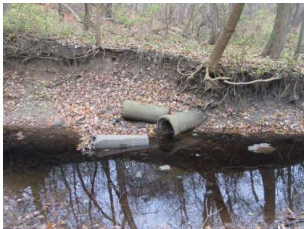
Erosion can damage infrastructure, such as storm sewer pipes.
