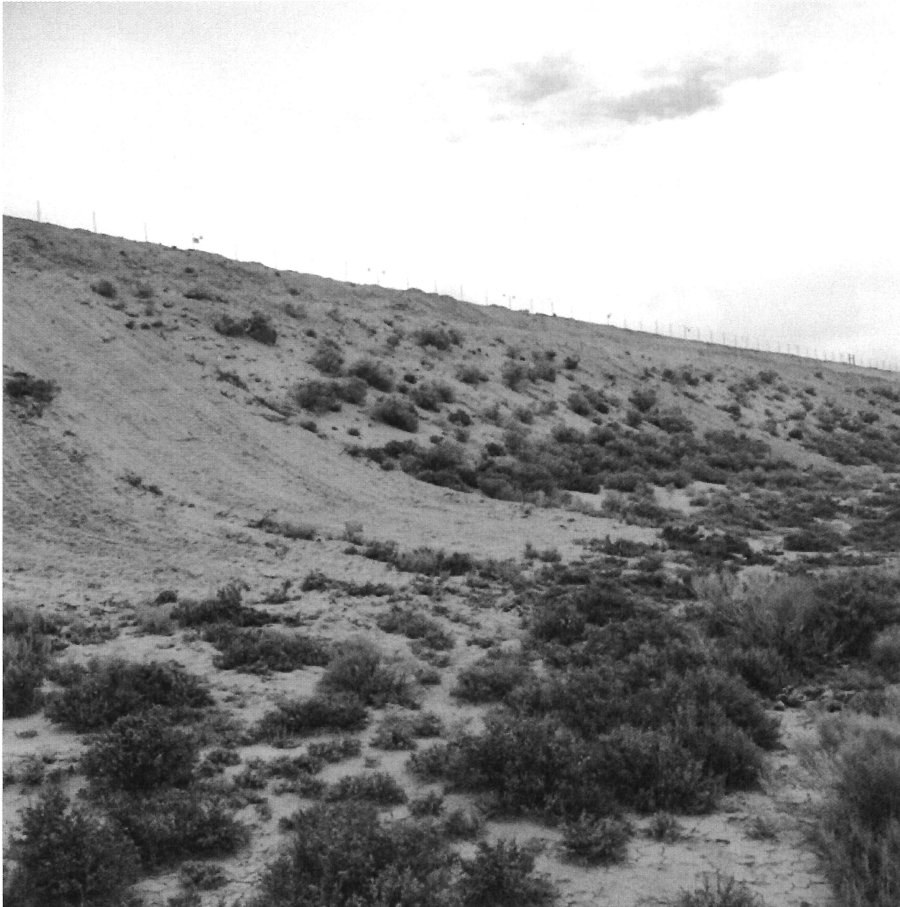
Photographs 2 Exterior of the south embankment. Note: Areas where rills were repaired on the embankment's outside slope with the bulldozer are visible on the left side of the image.
