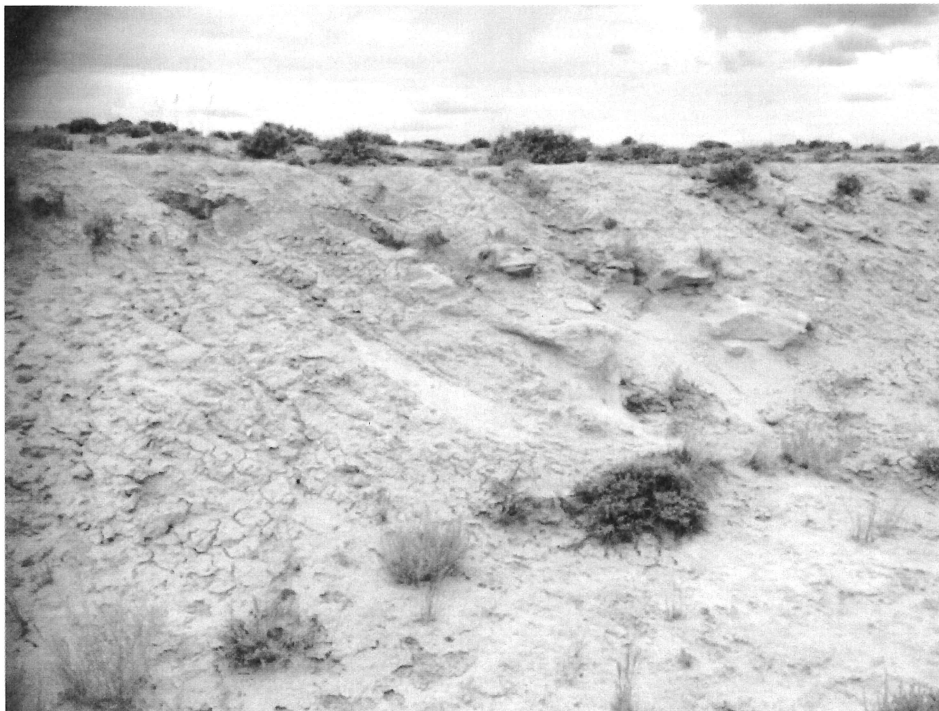
Photograph 6 Embankment rills, Reach 4/5, June 2014
