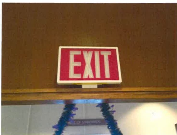
Figure 13- Generally licensed exit sign in Library
