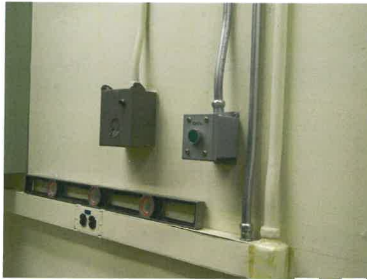
Figure 5 - Emergency stop button in vertical ranges in Rooms [REDACTED] and [REDACTED]
