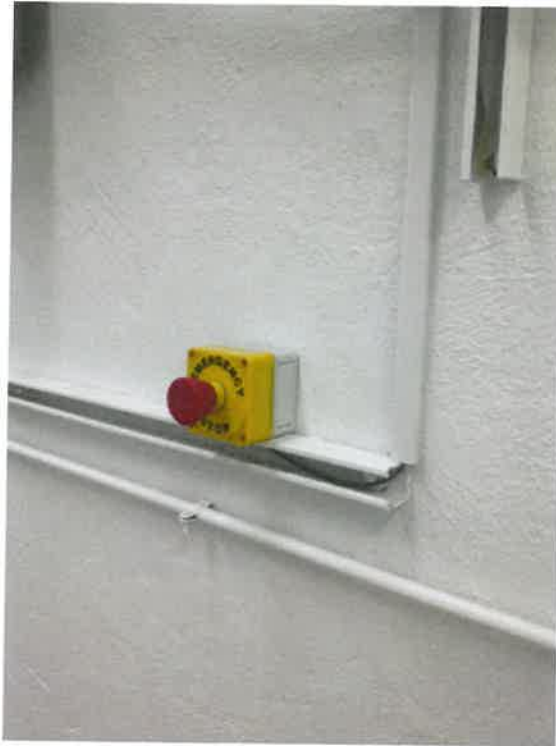
Figure 6 - Emergency stop in horizontal range Room [REDACTED]
