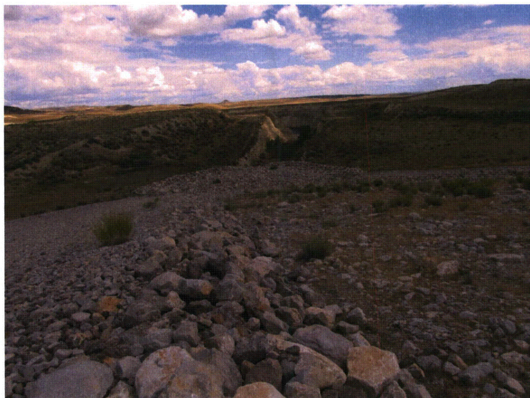
MAW 8/2014. PL-6. Diversion Channel No. 1 outlet into launch rock erosion protection basin on east side slope of disposal cell (Rob Pit in the background).
