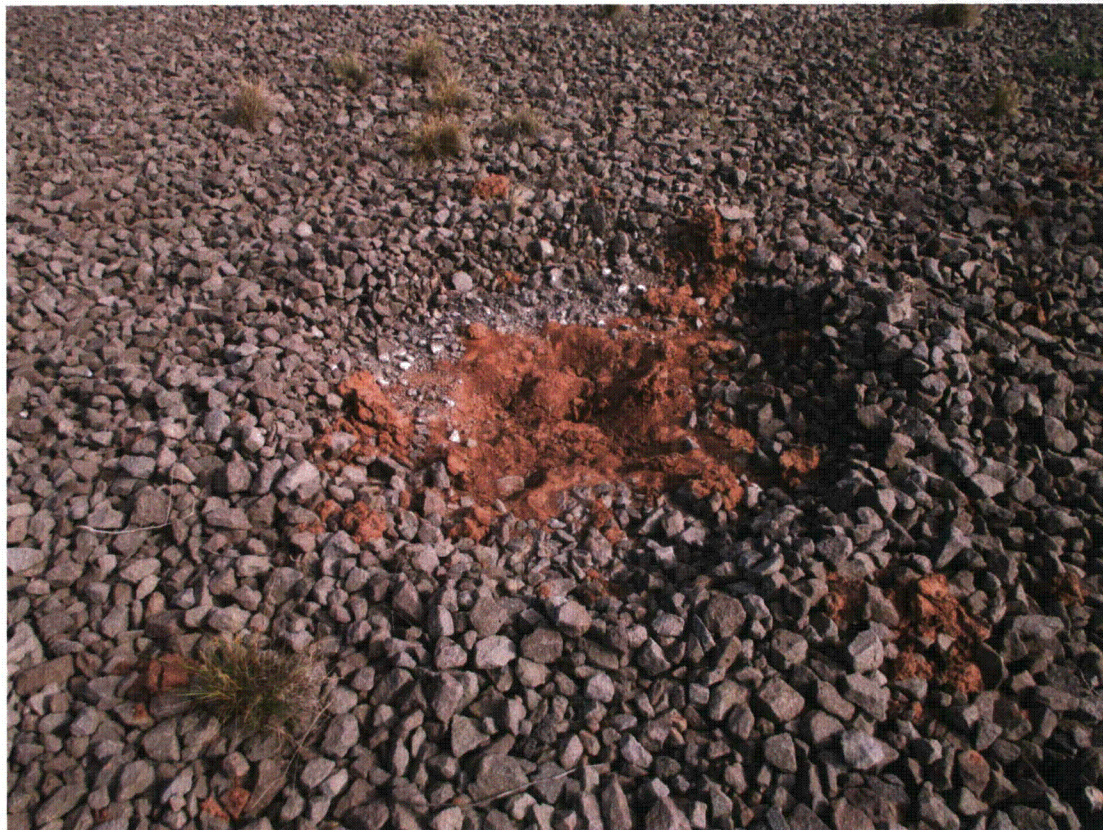
BLU 8/2014. PL-10. Exposed radon barrier surface on carbonate tailings disposal cell top slope.
