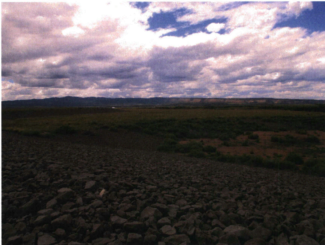
BLU 8/2014. PL-6. Acid tailings disposal area adjacent to main tailings disposal cell.
