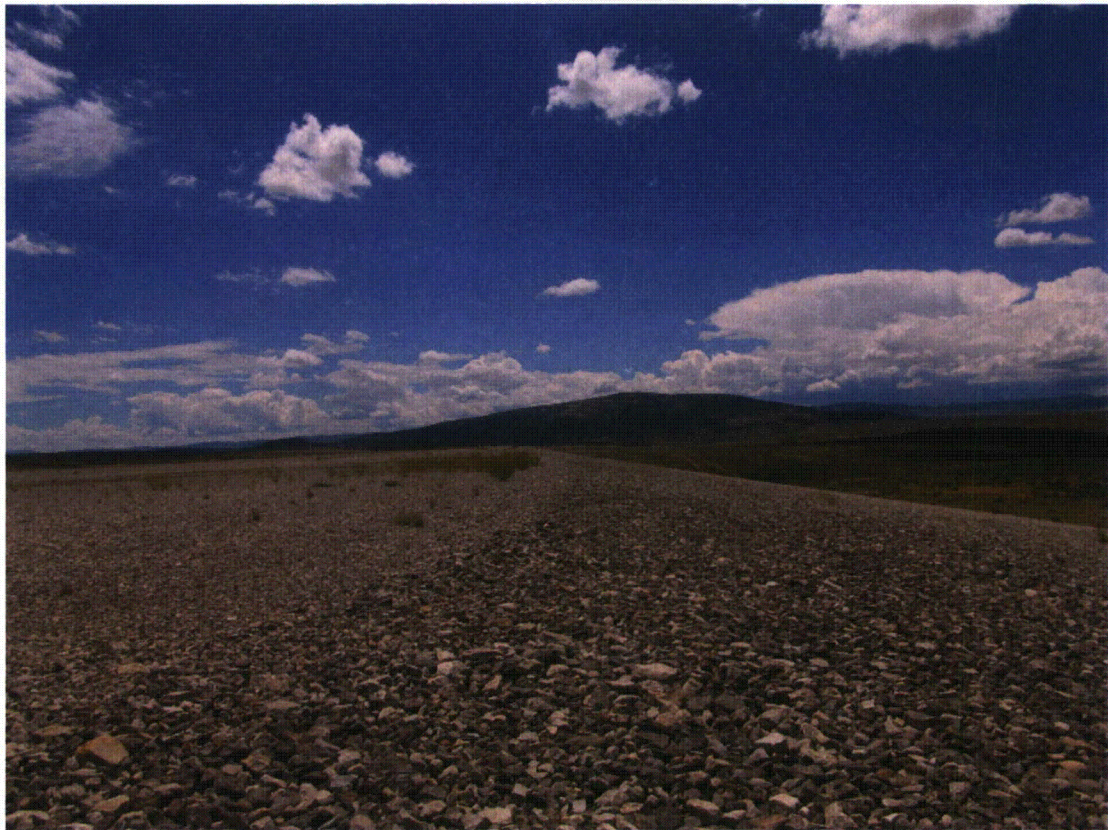
MAW 8/2014. PL-8. Intersection of west side slope and top of disposal cell.
