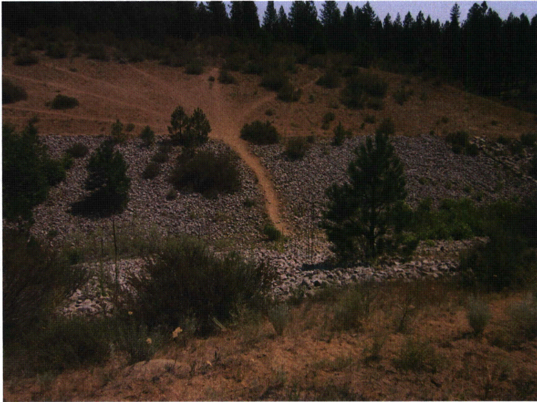
SHE 7/2014. PL-7. Displaced riprap along animal trails in diversion channel.
