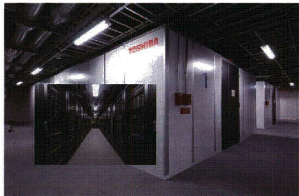
Cloud & Solutions Company, Data Center Image
