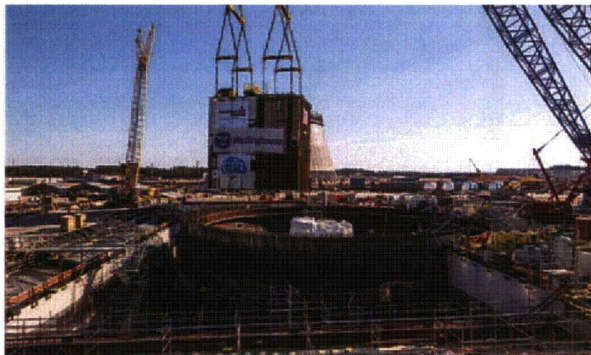
©2014 Georgia Power Company All rights reserved Installation of the largest module of the AP1000™, under construction in the US
