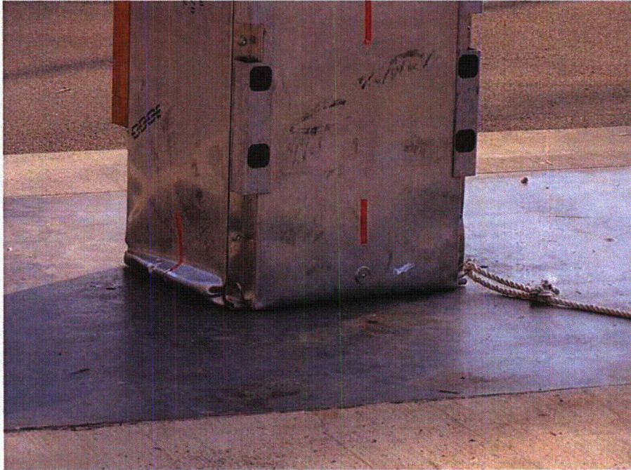
Figure 2-35 End Impact Damage (Top and Side)
