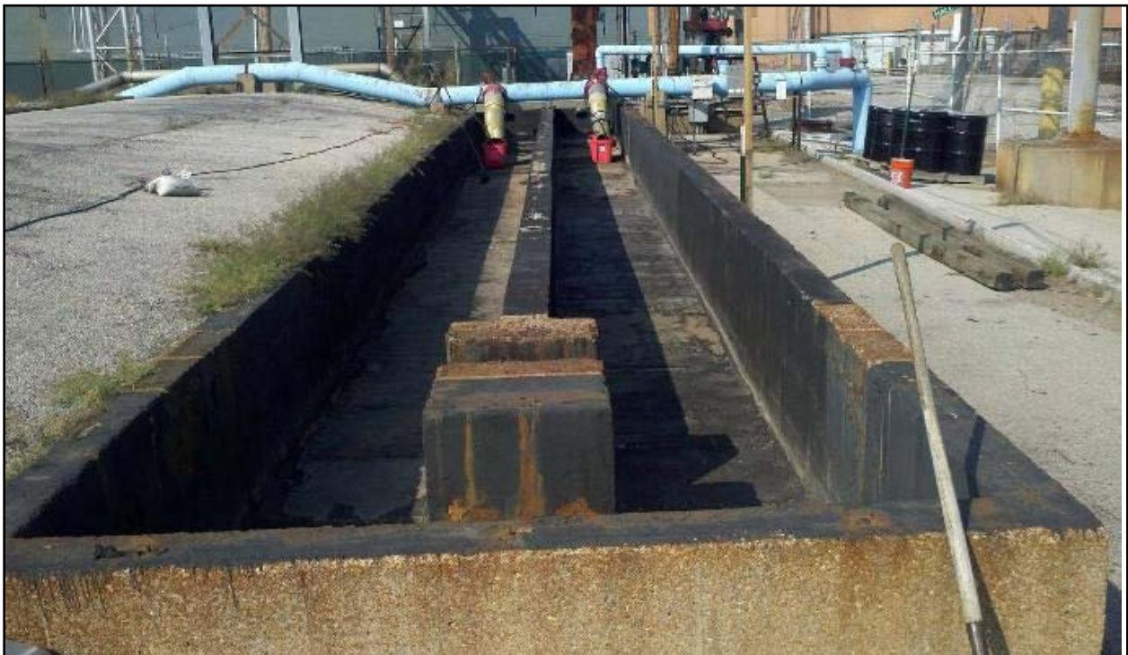
Figure 33-7 Photograph of Grit Chamber Looking West
