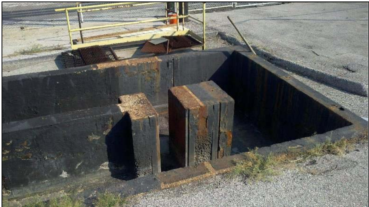
Figure 33-9 Photograph of East End of Grit Chamber Looking North
