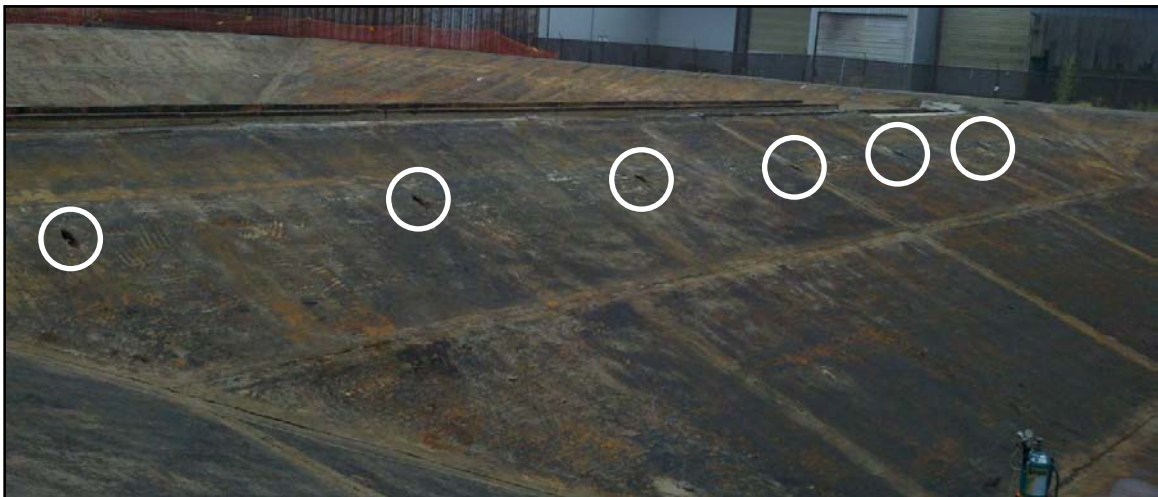
Figure 32-10 Photograph of West Basin Transfer Pipes
