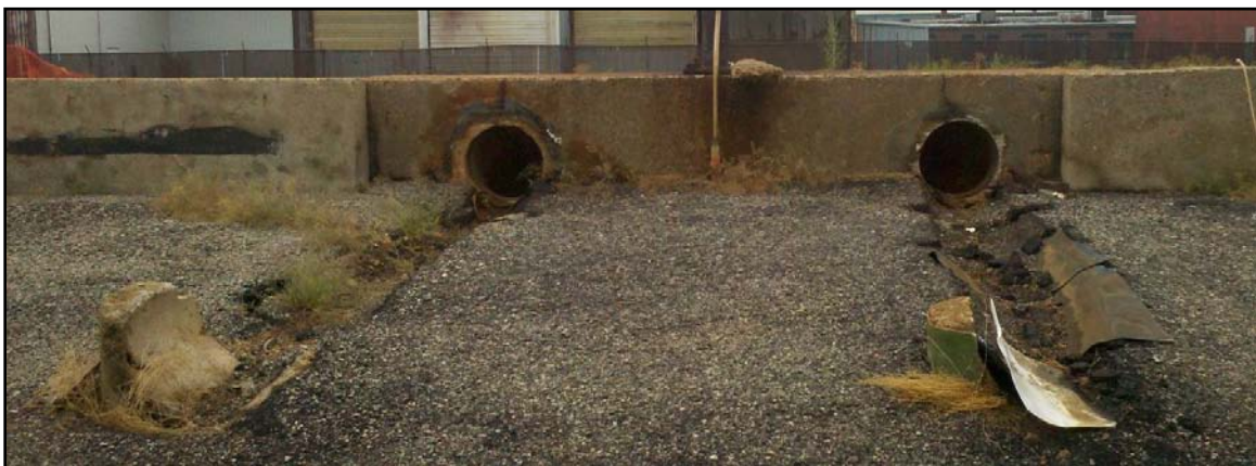
Figure 32-11 Photograph of West Basin Transfer Pipes
