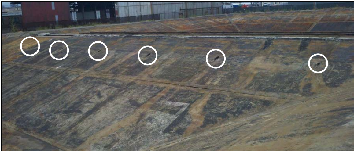
Figure 32-9 Photograph of East Basin Transfer Pipes
