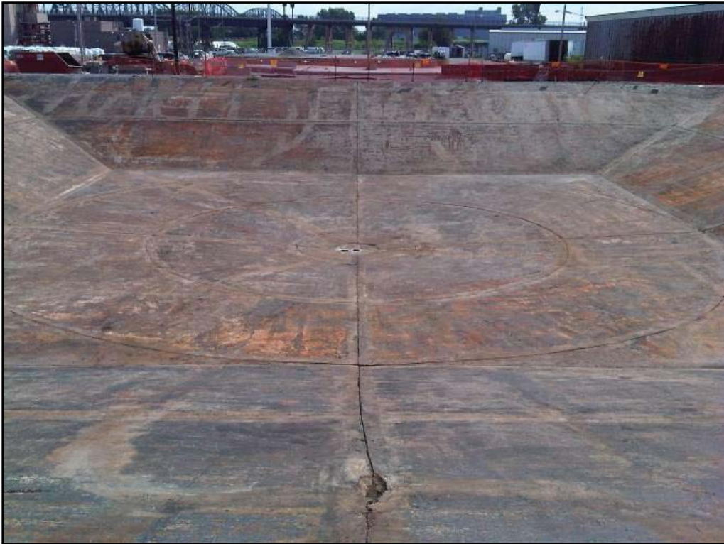
Figure 30-2 Photograph of Plant 7W East Basin Looking East
