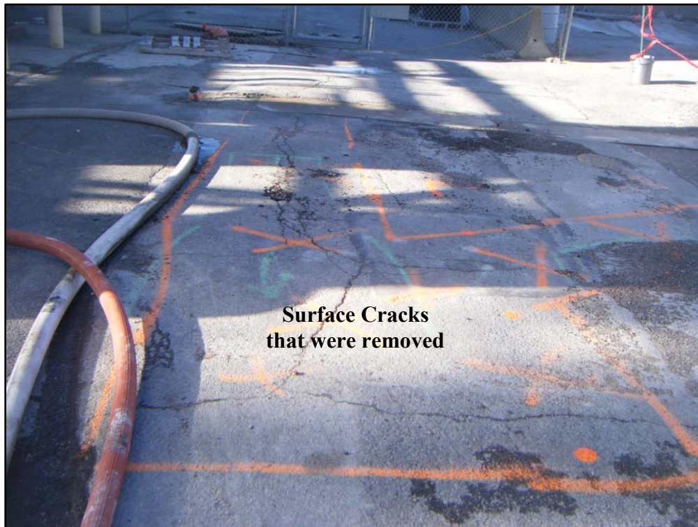
Figure 19-5 Photograph (3) SU13 Surface Cracks Removed
