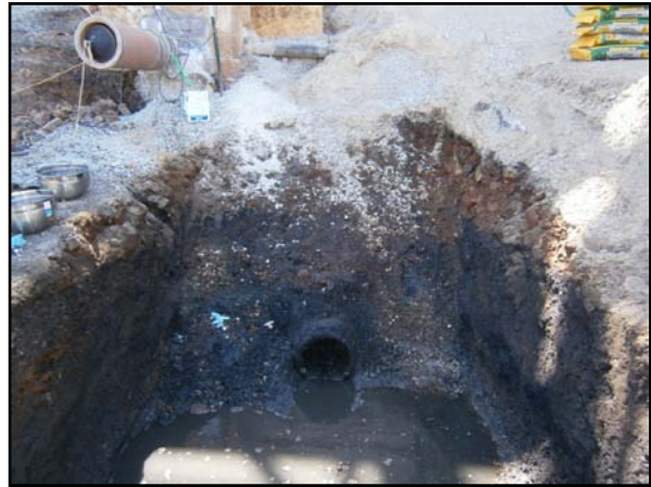
Figure 12-4 Photograph Looking West at the Terminus of the VCP Prior to Grouting
