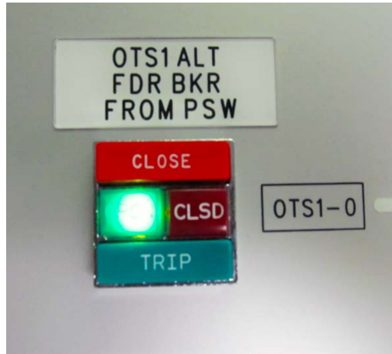
Breaker Switch on SSF Control Panel
