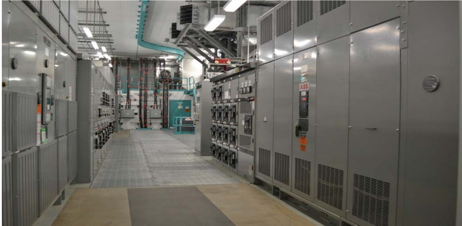
PSW Building Switchgear
