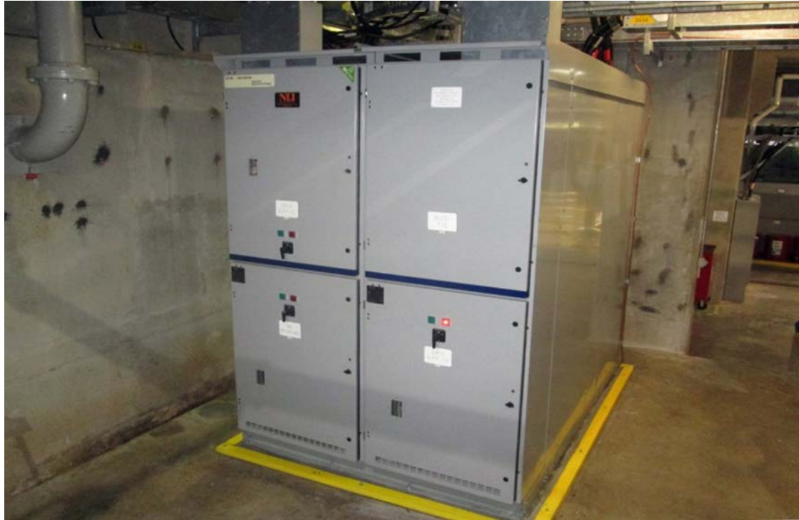
Keowee Switchgear Cabinet
