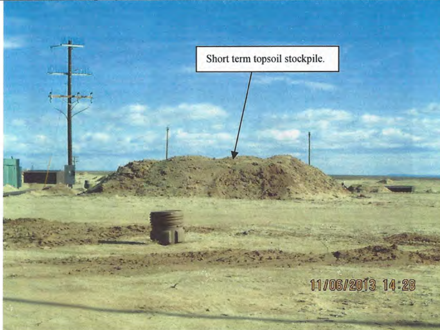
Photo Number 15: Short term topsoil stockpile in Mine Unit 1. The site's short term topsoil stockpiles must be inventoried and reported in the Annual Report.
