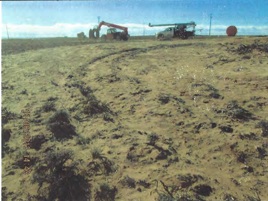
Photo Number 3: This depicts the toe ditch at the south end of topsoil stockpile #6. It is in constant need of maintenance due to its proximity to the road leading to the Plant Site.
