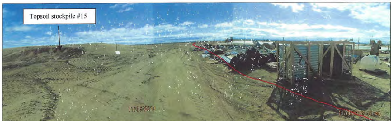
Photo Number 26: This depicts the pond diversion ditch just north of the ponds. The ditch runs east-west here. This view is looking east and it depicts equipment being stored in the ditch's channel (red line). This is unacceptable and the equipment must be removed immediately. LCI staff will need to cordon-off the ditch's path at this location to prevent unwanted equipment storage at this location in the future. Topsoil stockpile #15 is on the left side of this photo. Materials had recently been removed from topsoil stockpile #15, which explains the recent scar indicated by the black arrow in this photo. A more well-defined toe-ditch will need to be created along the flank of topsoil stockpile #15.
