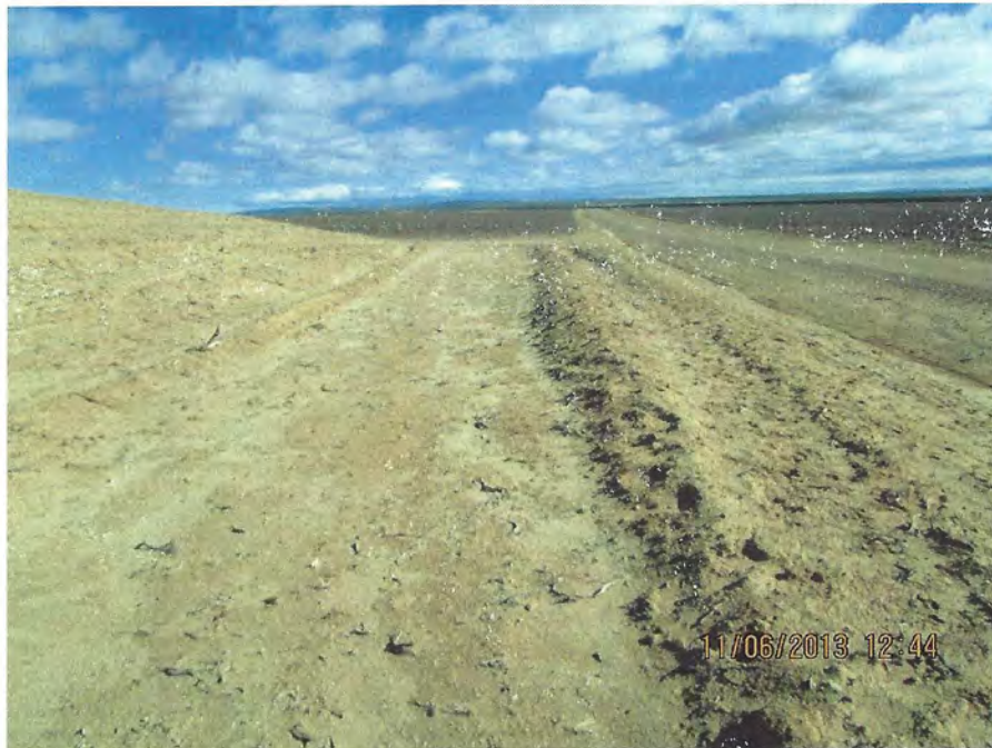
Photo Number 8: This depicts the toe-ditch around topsoil stockpile 3. It is in good condition here but is in need of some extra definition in some locations.
