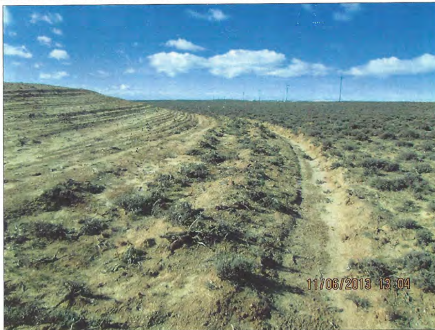
Photo Number 9: This depicts the toe ditch at the northwest corner of topsoil stockpile #4.
