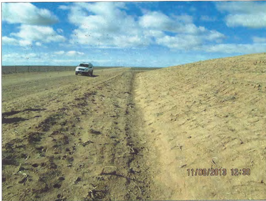
Photo Number 5: This depicts the toe ditch on the south face of topsoil stockpile #2. This view is looking west. The LCI project's access road is on the left side of this photo. This ditch is in good condition.
