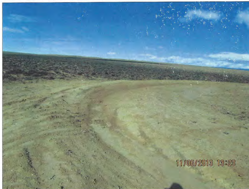
Photo Number 11: This depicts the toe-ditch around topsoil stockpile #8. It is an exemplary ditch around the entire perimeter of the stockpile. This view is looking toward the northwest. Note the accumulation of coarse grained sands on the surface. This is due to the winnowing of finer materials from the topsoil due to wind erosion.
