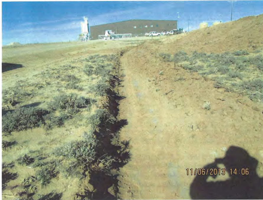
Photo Number 29: This is a view looking north along the west flank of topsoil stockpile #6. The toe ditch here was also recently reestablished.
