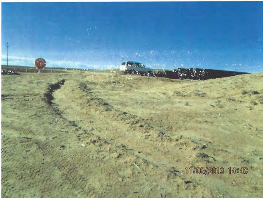
Photo Number 4: This depicts the toe ditch in the south end of the topsoil stockpile at DDW-4.
