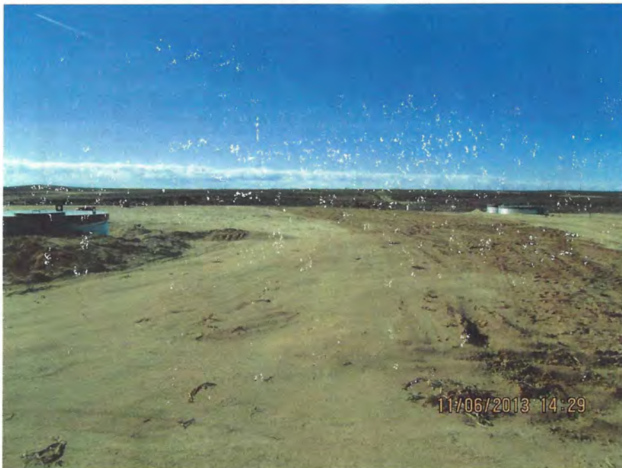
Photo Number 16: This depicts an area at the northwest corner of MU1 where some topsoil has been respread adjacent to a proposed travel route. Care must be taken in these scenarios to ensure topsoil is not trampled once it is reapplied.
