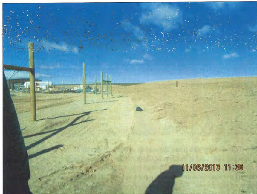
Photo Number 24: This is a view looking north along the diversion ditch that runs along the east side of the ponds. There are no concerns with the ditch's construction. Some trash is evident in the middle of the photo.
