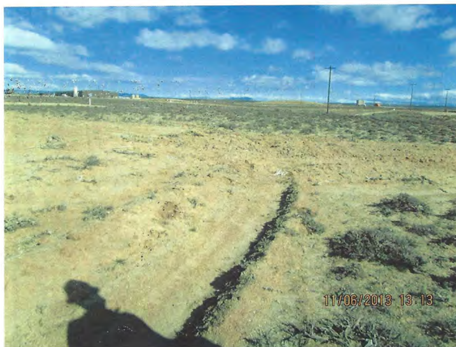
Photo Number 10: This depicts the east end of the toe ditch around topsoil stockpile #5. This area needs to be redefined. View is looking northeast.
