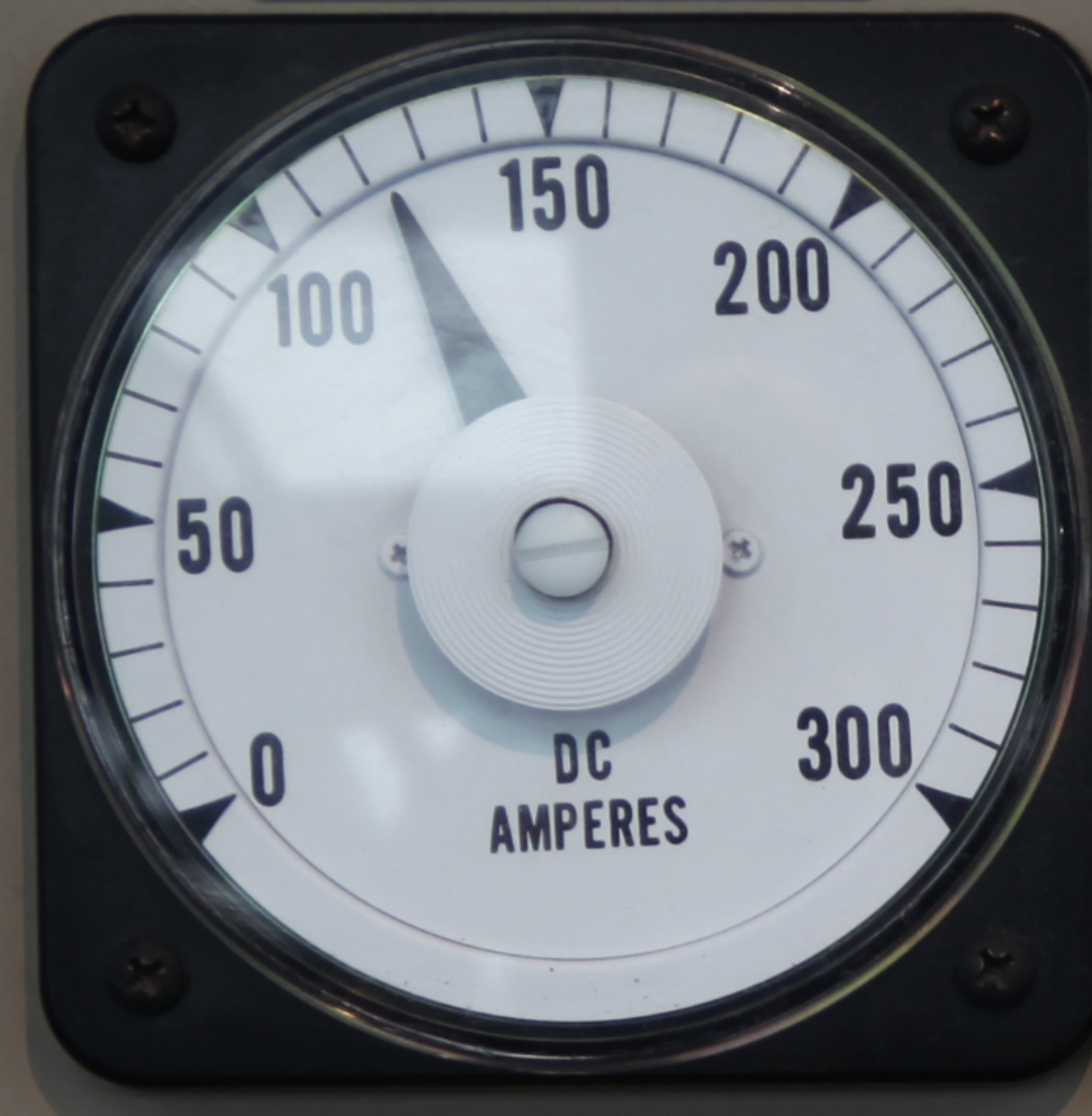
DIESEL GENERATOR B FIELD PEB-II-G02F
