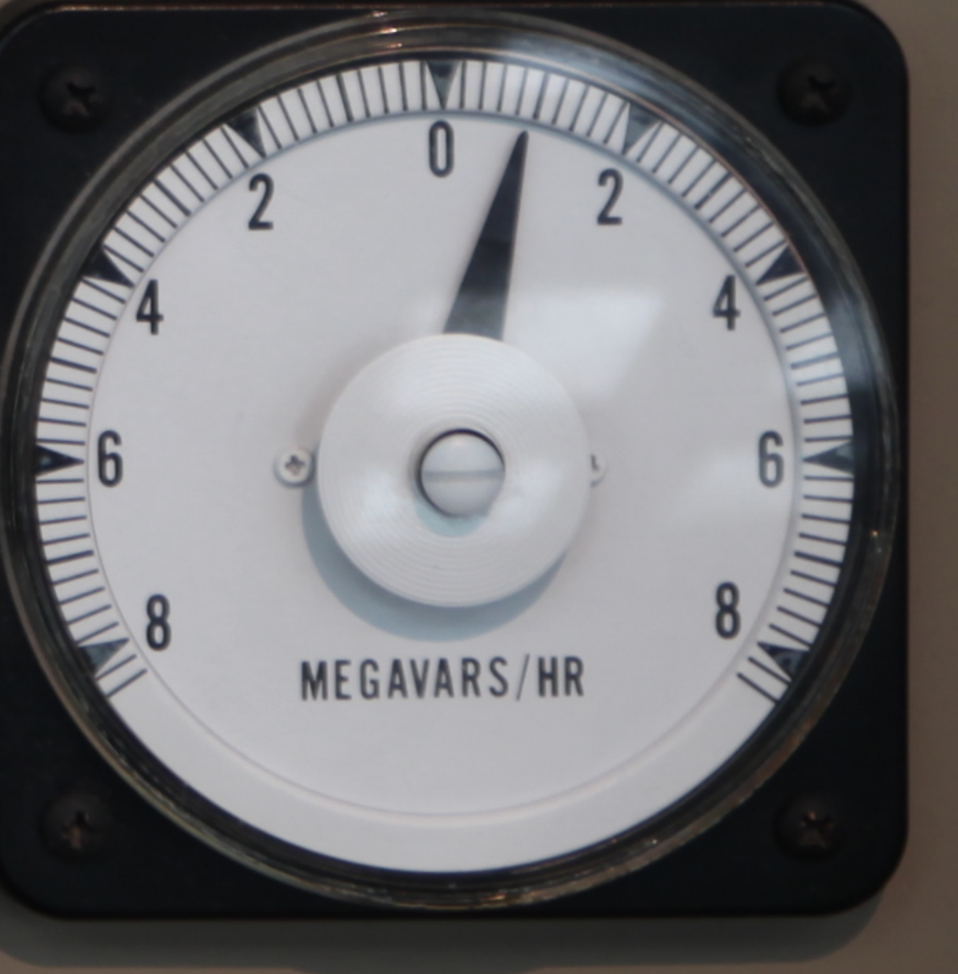
DIESEL GENERATOR B G02 PEN-JIV-G02
