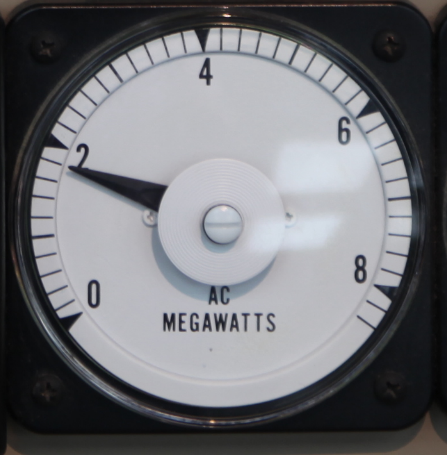
DIESEL GENERATOR B G02 PEN-JIW-G02
