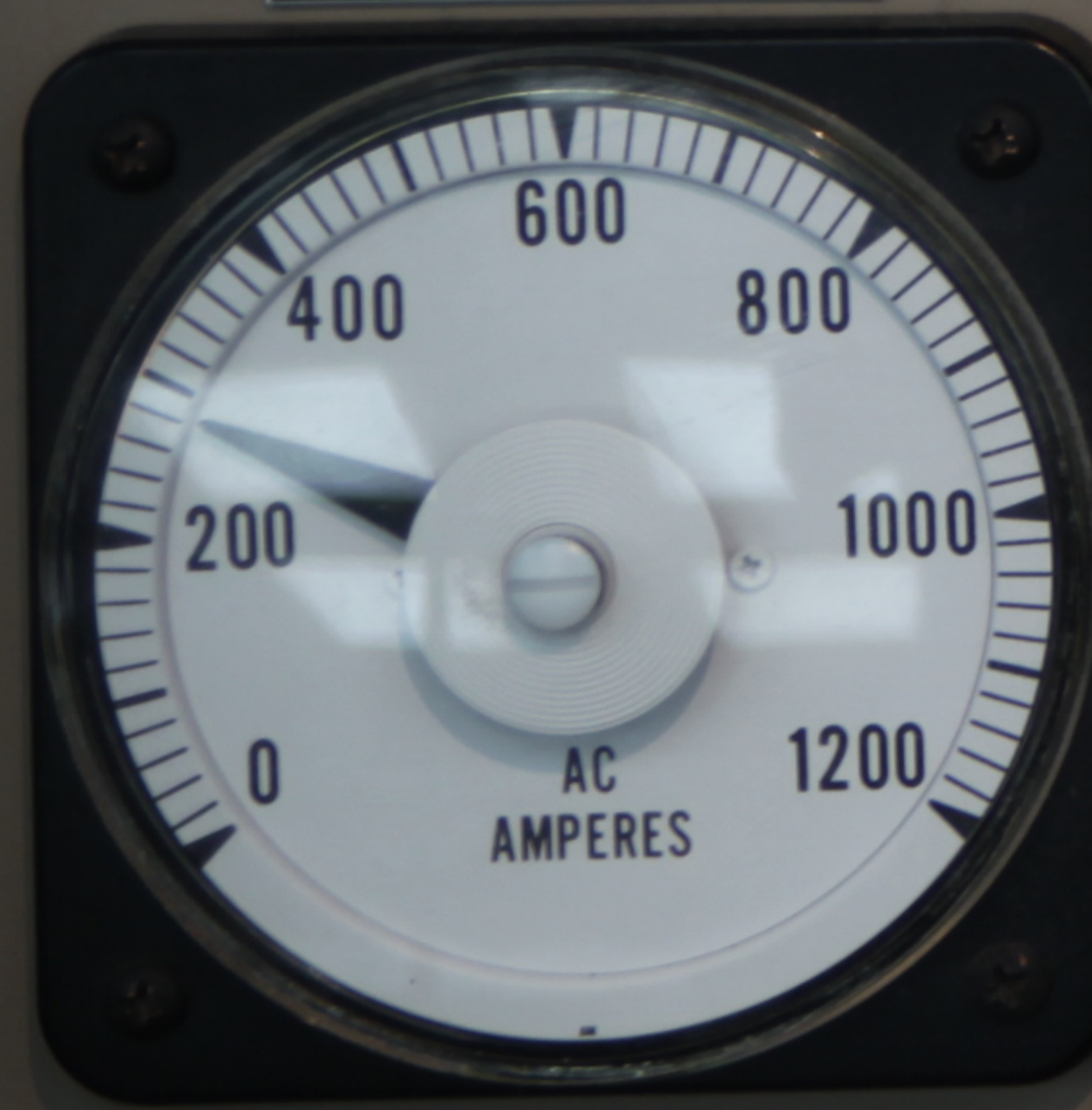
DIESEL GENERATOR B G02 PEN-II-G02
