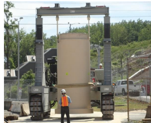
VCT transporting HI-TRAC and loaded STC from U3 to U2
