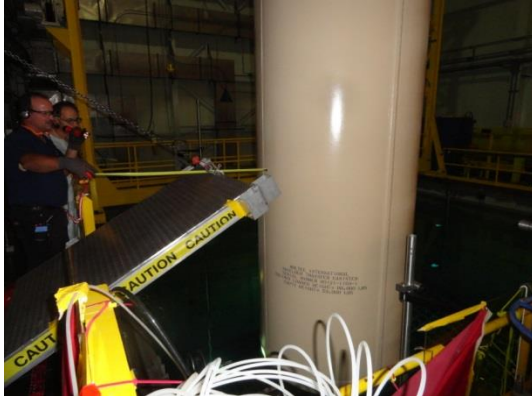
Empty STC going into U3 spent fuel pool
