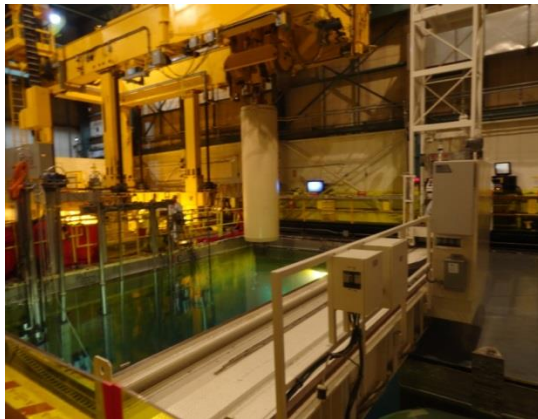
Loaded STC lowered into U2 spent fuel pool to be unloaded
