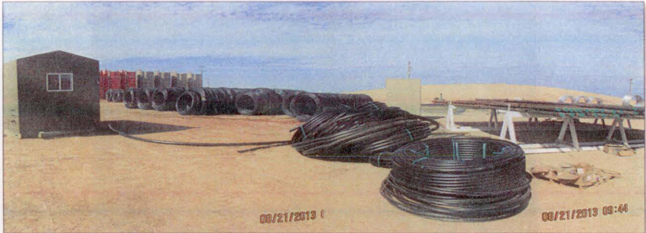
Photo Number 4: This depicts a portion of the DDW-4 drill pad where equipment that came from the "field laydown area" is now stored.
