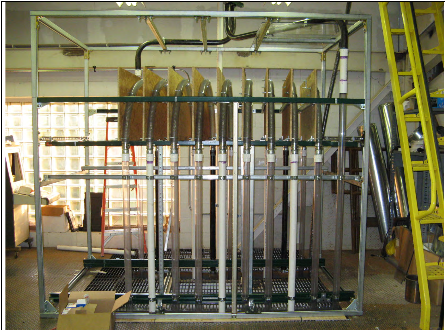
Figure 2-8 Vertical Cooling Coil Assembly, - Second Floor
