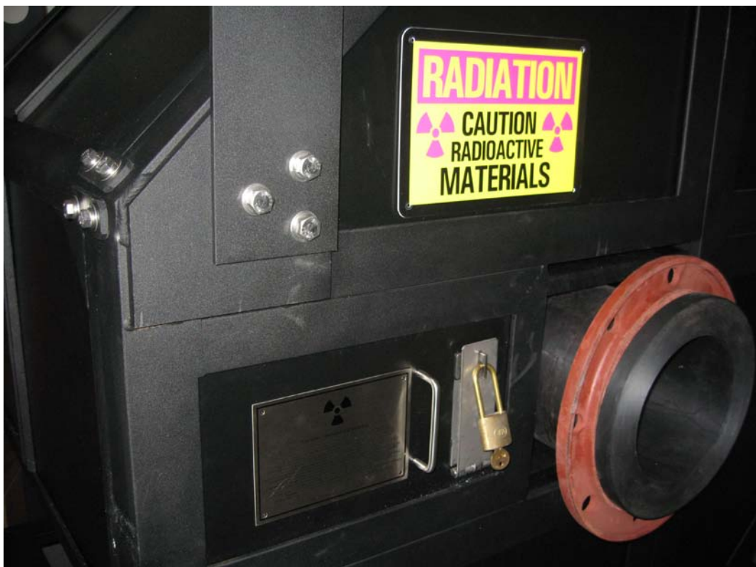
View of the SABIA X1-XP analyzer, showing the source access closed and locked. This unit was designed for operation with an 8 inch pipe (installed)
