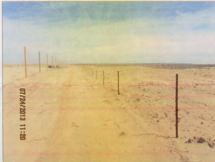
Photo Number 4: This is a view looking north along the diversion ditch that goes around the east edge of the Ponds in the Plant Site. It is to-grade and topsoil reapplication is in-progress.
