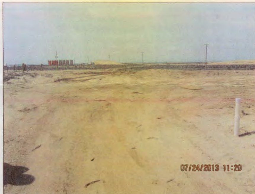
Photo Number 5: This is a view looking south along the diversion ditch that goes around the east edge of the Ponds in the Plant site. It is to-grade and topsoil reapplication is in-progress.
