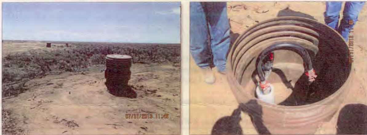
Photo Number 1: The photo on the left depicts the well cover for one of the HH 1-3 well inspected today. It is on the west edge of HH 1-3, west of a prominent drainage (which is behind this well). The wells in HH 1-3 are at least 20 feet away from the drainage. The photo on the right depicts the inside of the well depicted on the left. It is currently set up with injection well hardware.
