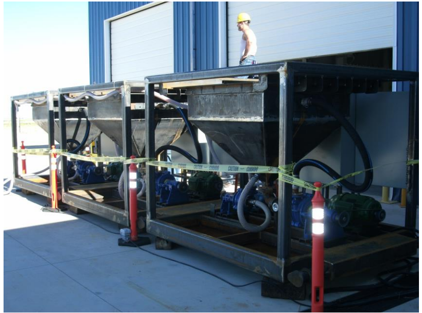
Figure 1 – Initial hydraulic flow tests being undertaken on the 3 x interconnected Ablation modules that will comprise part of the 5tph Ablation Unit that is nearing completion.
