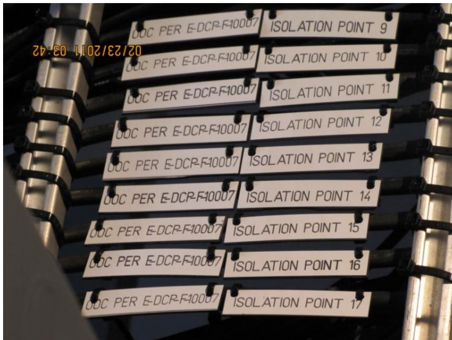
Figure 3.1-2: Electrical Isolation at an Electrical Control Room
