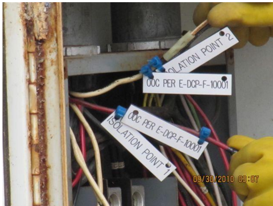
Figure 3.1-3: Electrical Isolation at Lighting Panel
