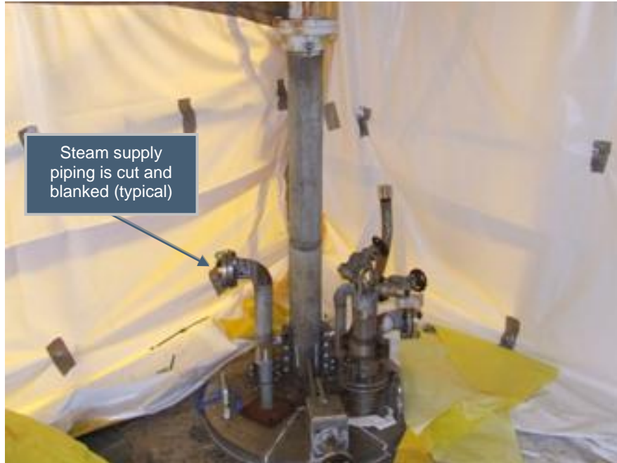
Figure 3.1-1: Transfer Jet Isolated from the Steam System (Tank 19)
