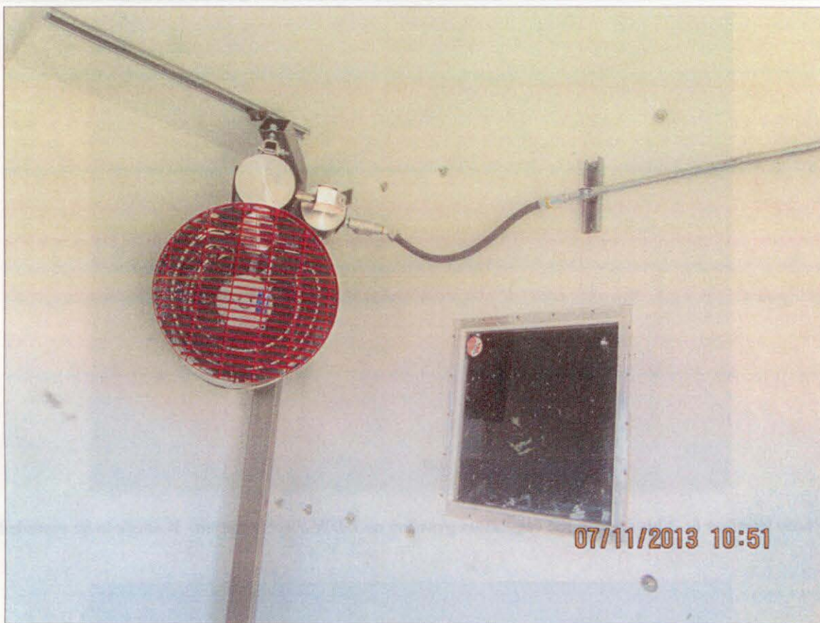
Photo Number 4: This depicts the heater inside the DDW-1 pump house.
