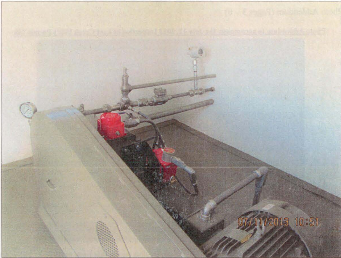
Photo Number 3: This depicts the pump housed in the DDW-1 pump house.
