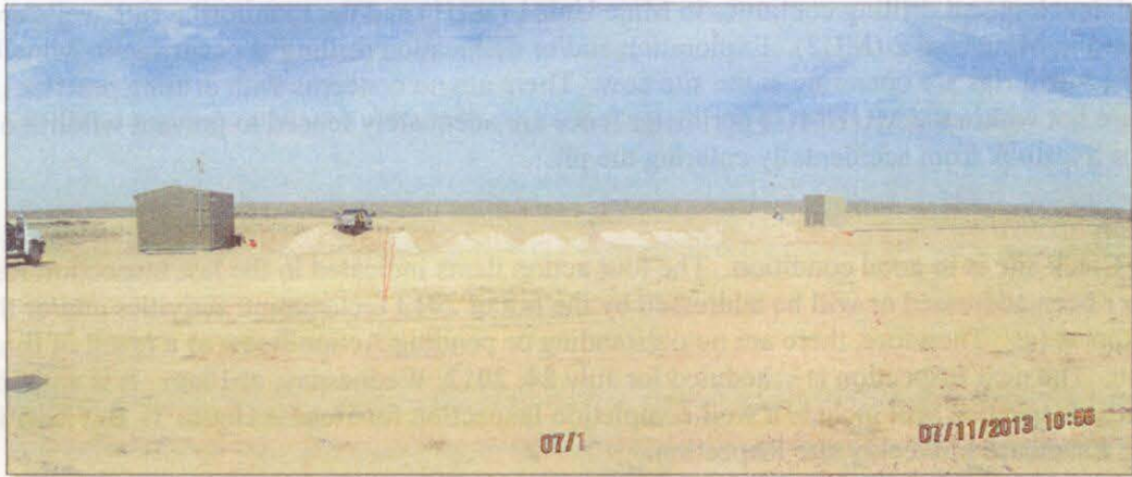
Photo Number 2: This depicts the pump house (structure on left) and well head cover (structure on right) at Deep Disposal Well 1 (DDW-1). The trench between the two structures was open during this Inspection, as piping was being installed. This view is looking west.
