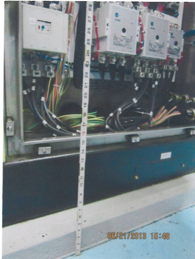
Interior of K-3A control cabinet
