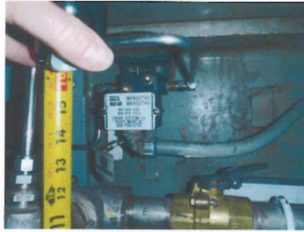
EDG starting air solenoid valve (typical)
