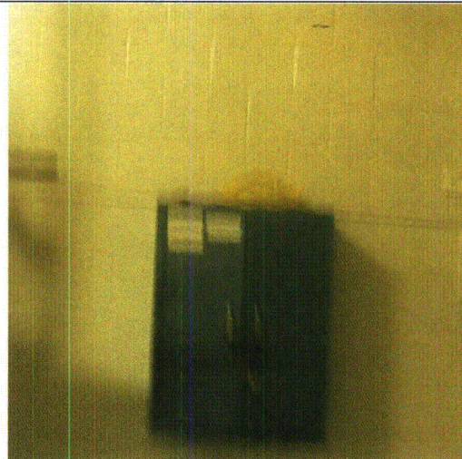
Note: Unrestrained cable and tools on top of the operations equipment cabinet
