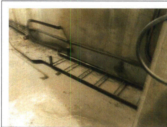
Note: unrestrained ladder by the north wall.
