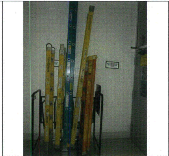
Note: Unsecured ladders at the Nonregenerative heat exchanger room
