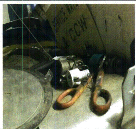
Note: Tools on top of CCW tank
