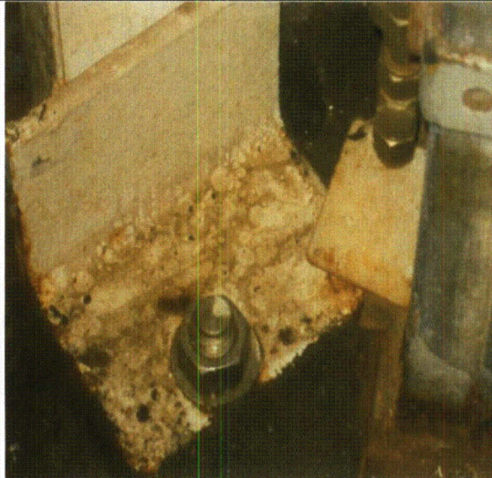
Note: Anchor bolt for strainer (stainless steel) with some corrosion of base angle.
