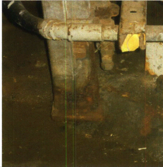
Note: Corrosion at the base of a Unistrut column
