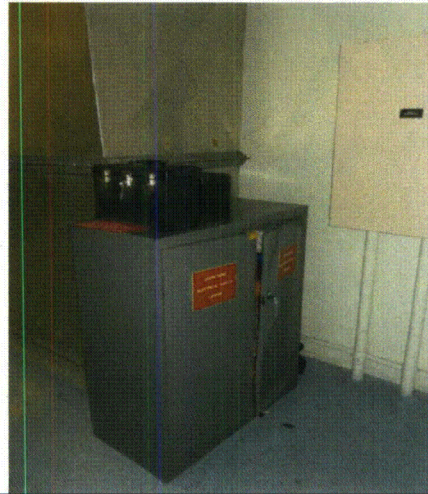
Note: Unsecured tool box on top of cabinet and cabinet door not closed.
