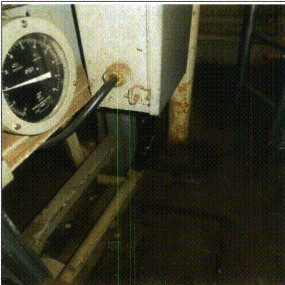
Note: Pipe support stanchion showing considerable corrosion
