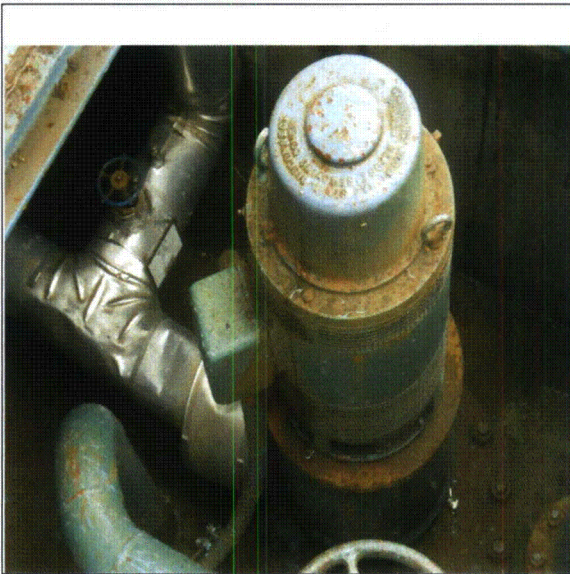
Note: F.O. Transfer Pump
