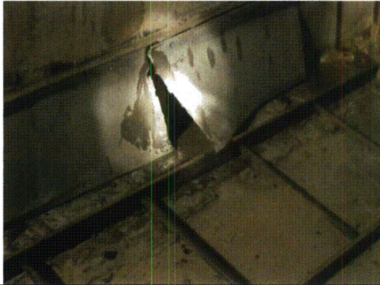
Note: Broken flashing
