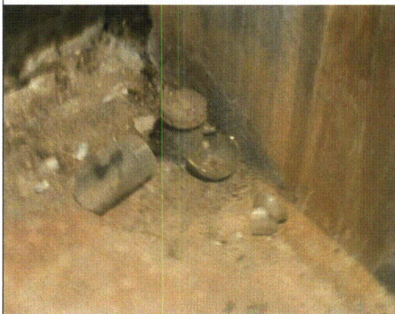
Note: Broken glass in the east corner of the room.
