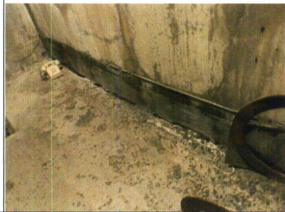
Note: Missing flashing along the wall
