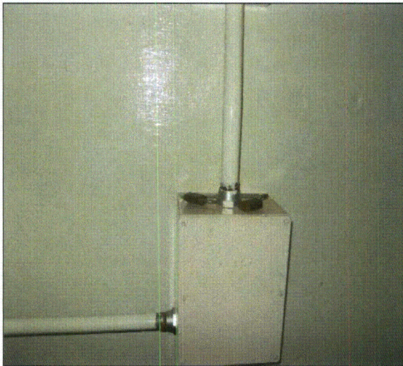
Note: Loose padlocks on top of cabinet
