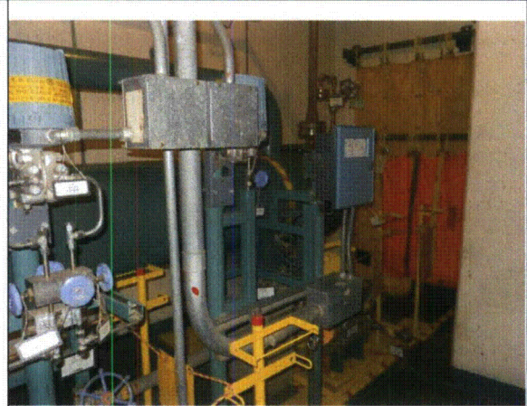
Note: View of equipment and conduits
