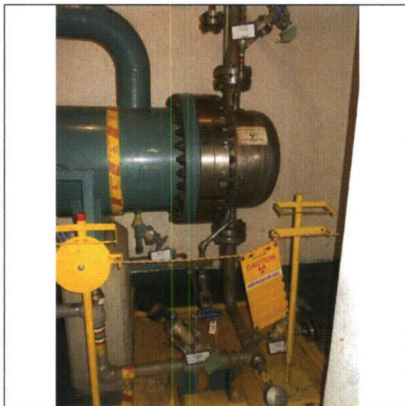
Note: View of removeable exchanger head
