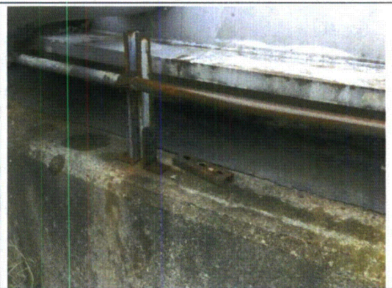
Note: Loose Unistrut on top of RWST-31 foundation.
