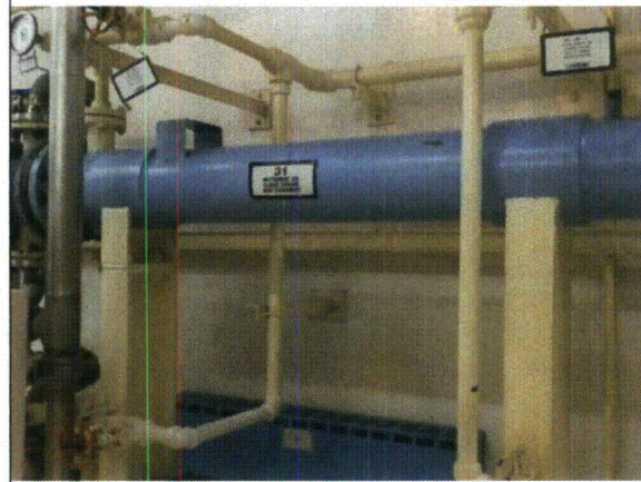
Note: Exchanger 31 mounted above Exchanger 32
