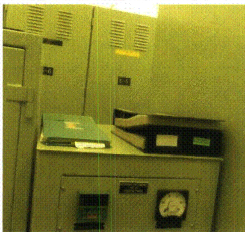
Note: unrestrained binders on top of Hydrogen Recombiner No. 31 Control Panel
