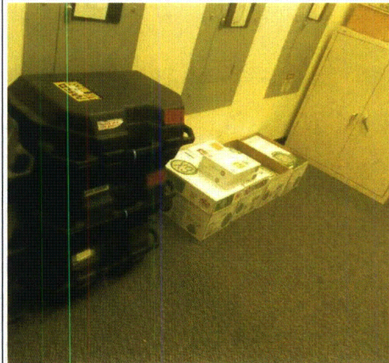
Note: Boxes against the west wall on the floor and a box resting on top of a cabinet at the northwest corner of the room
