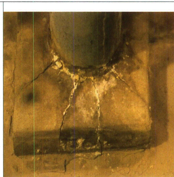
Note: Cracked grout penetration protection
