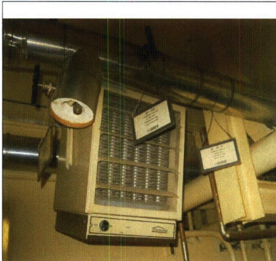
Note: Pipe insulation interference with heater.
