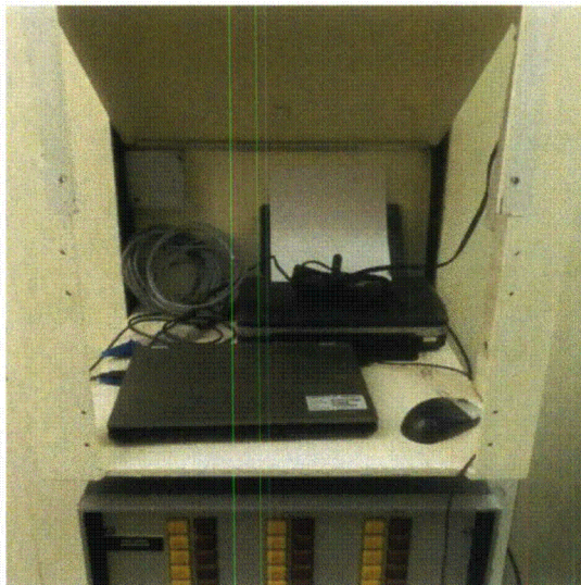
Note: Rack adjacent to Instrument Bus 31 has an unrestrained laptop and printer
