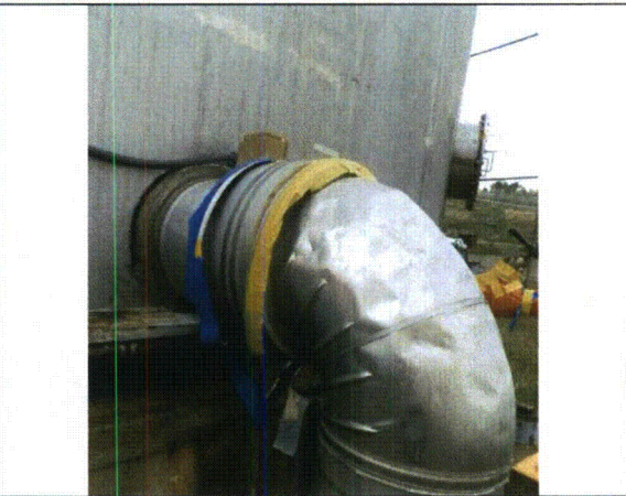
Note: Piping insulation connection held with tape.
