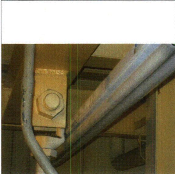
Note: One of the florescent fixtures is touching the steel hanger.
