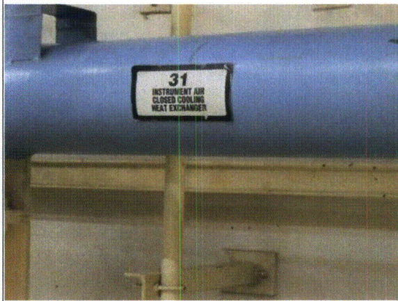
Note: Exchanger 31 mounted above Exchanger 32
