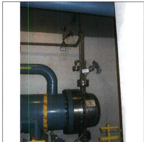
Note: View of exchanger removeable head
