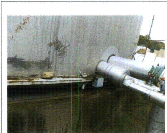
Note: Rock resting on the tank ring.
