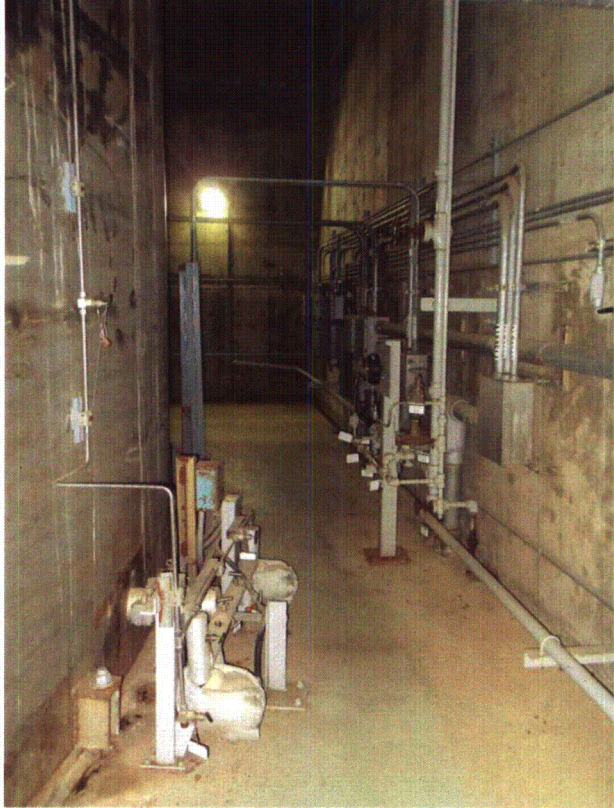
Area # Yard, 45, CAL-TKFROOM 8-15-12 006
