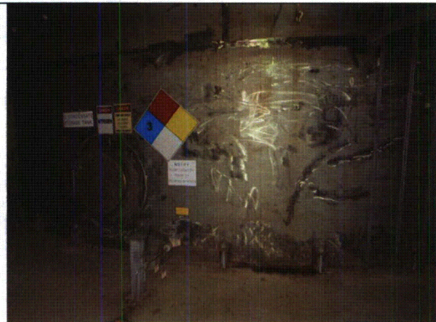
Area # Yard, 45, CAL-TKFROOM 8-15-12 004
