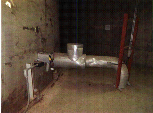
Area # Yard, 45, CAL-TKFROOM 8-15-12 008
