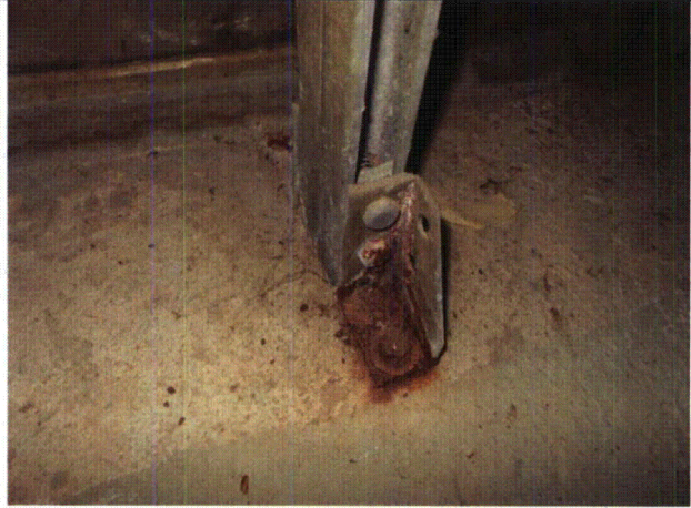
Area # Yard, 45, CAL-TKFROOM 8-15-12 014
