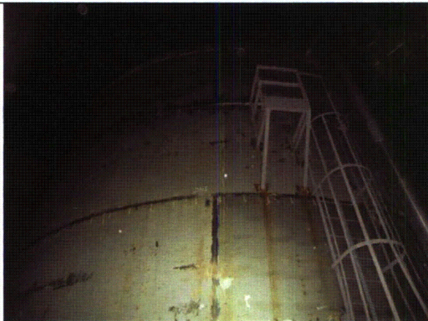
Area # Yard, 45, CAL-TKFROOM 8-15-12 003
