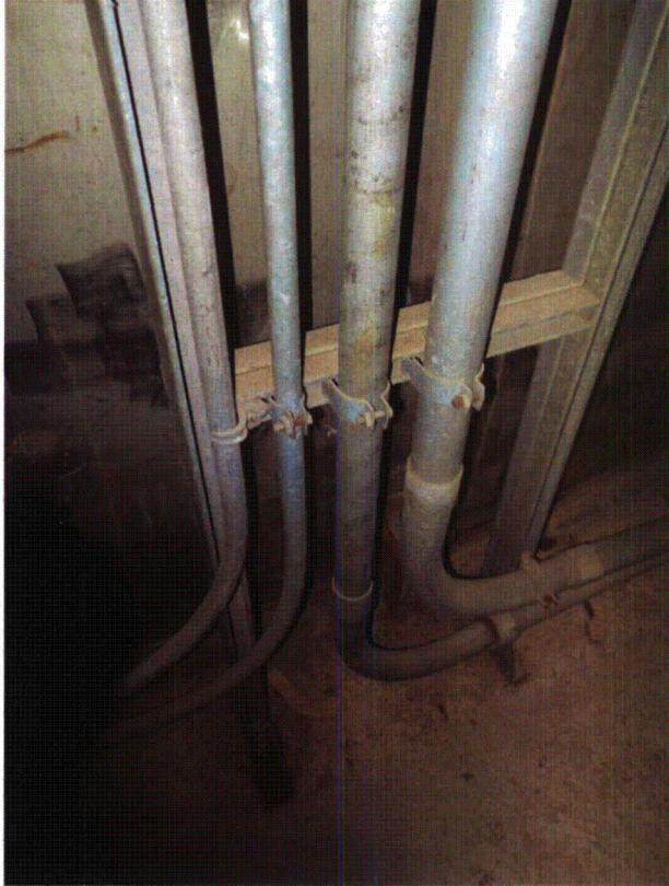
Area # Yard, 45, CAL-TKFROOM 8-15-12 013
