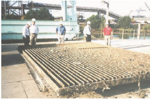
Intake Trash Bars
