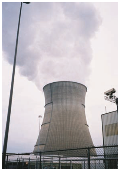
Natural Draft Cooling Tower
