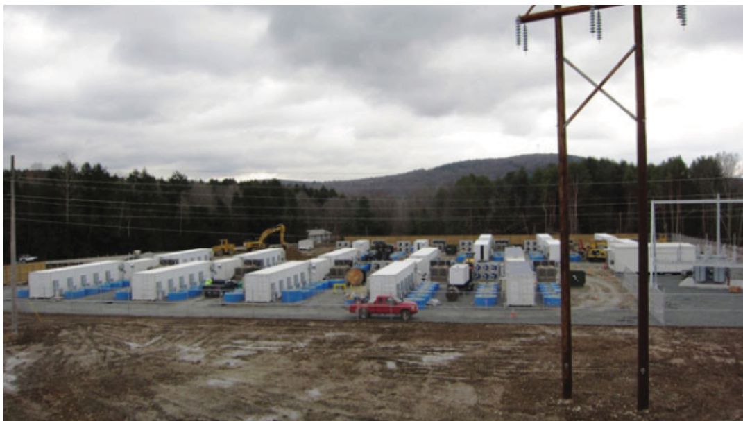
Beacon Power's Stephentown, N.Y., storage plant during construction. The blue cylinders on the ground are the flywheels.
