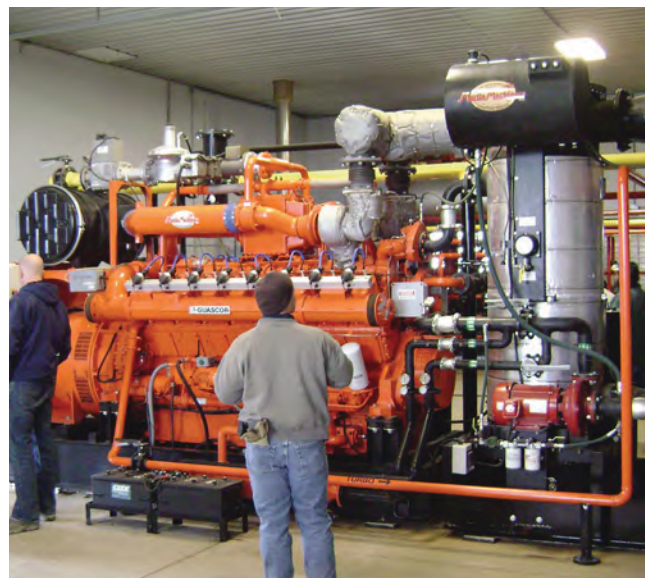
Biogas Generator – NYSERDA photo
